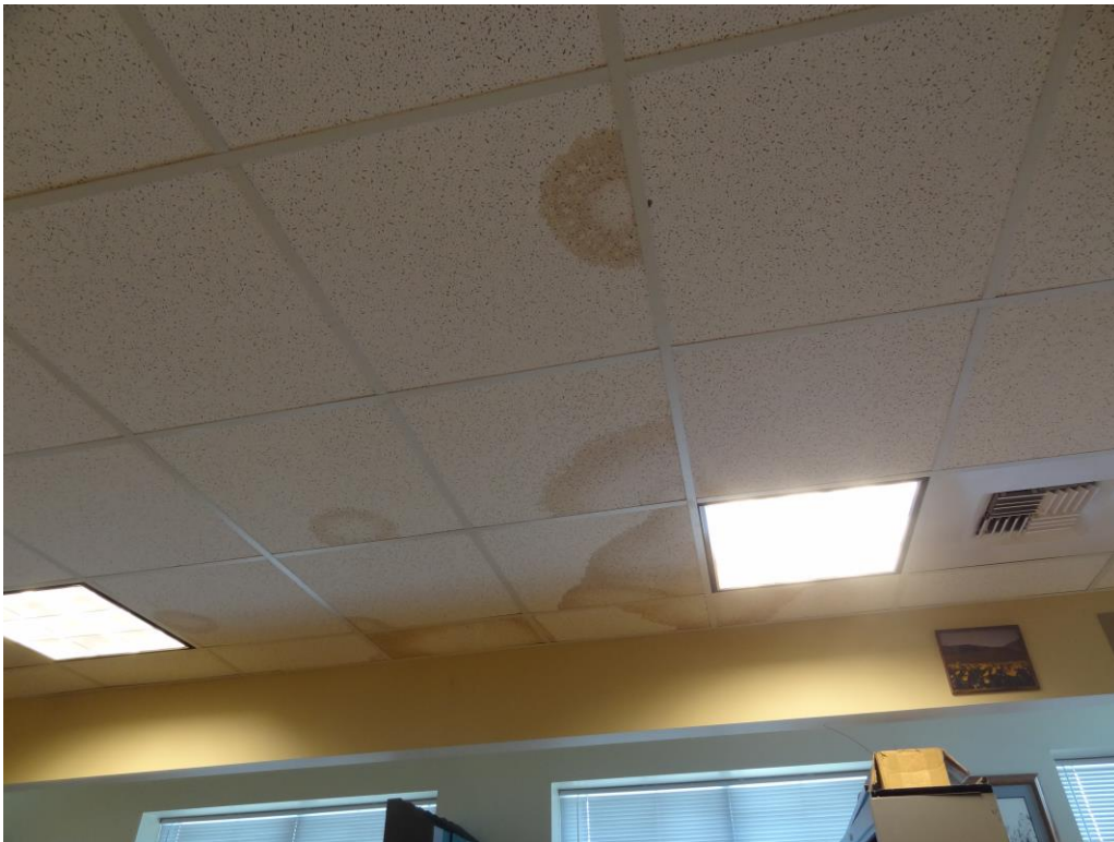
Elko Eastern Region Office - Building #2297 Description: Ceiling tile replacements needed.
