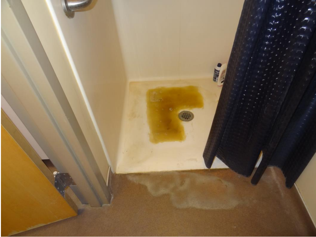
Elko Eastern Region Office - Building #2297 Description: ADA shower upgrade needed.
