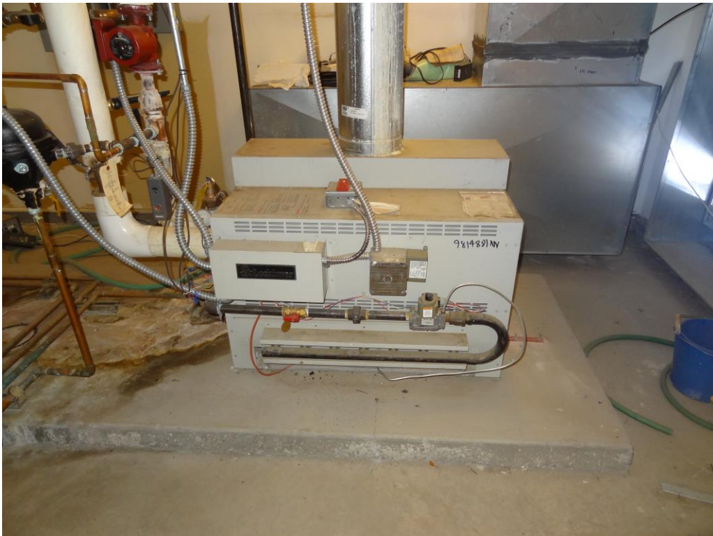
Elko Eastern Region Office - Building #2297 Description: Boiler replacement needed.
