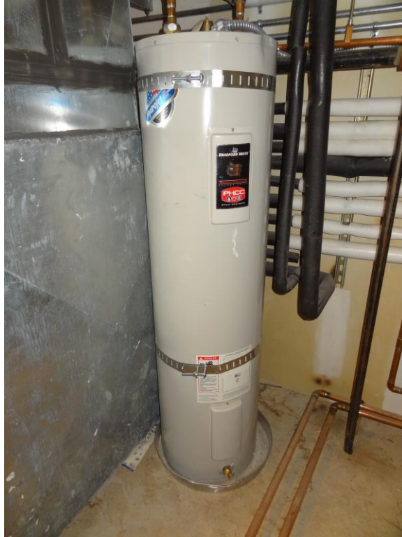
Elko Eastern Region Office - Building #2297 Description: Water heater replacement needed.
