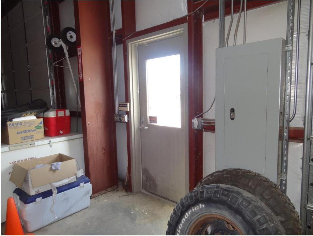
Elko Eastern Region Garage - Building #2298 Description: Clearance at electrical panel needed.
