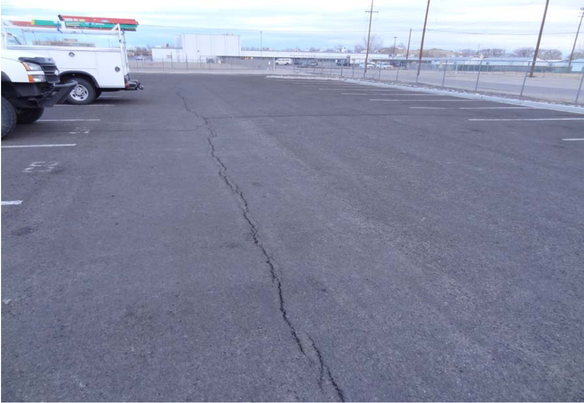
Fallon National Guard Armory Site - Site #9885 Description: Paved parking area in need of crack filling.
