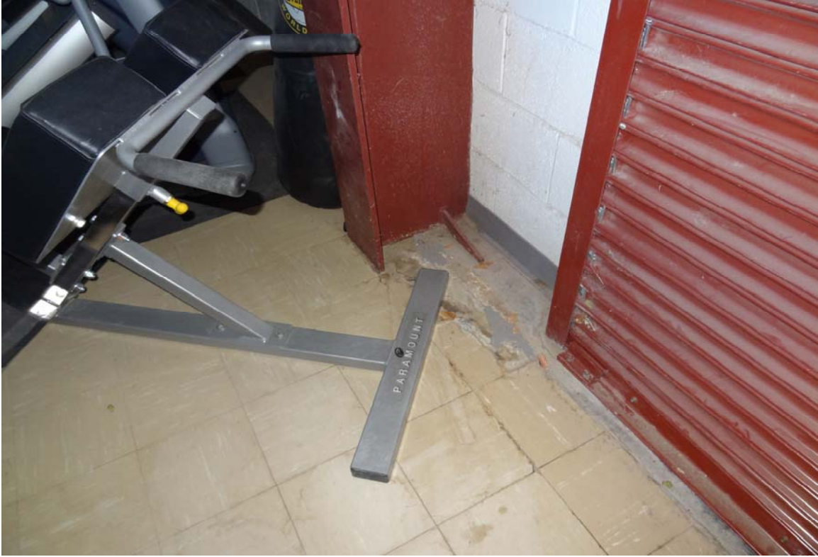
Fallon Armory - Building #0678 Description: Damaged VCT in Gym.
