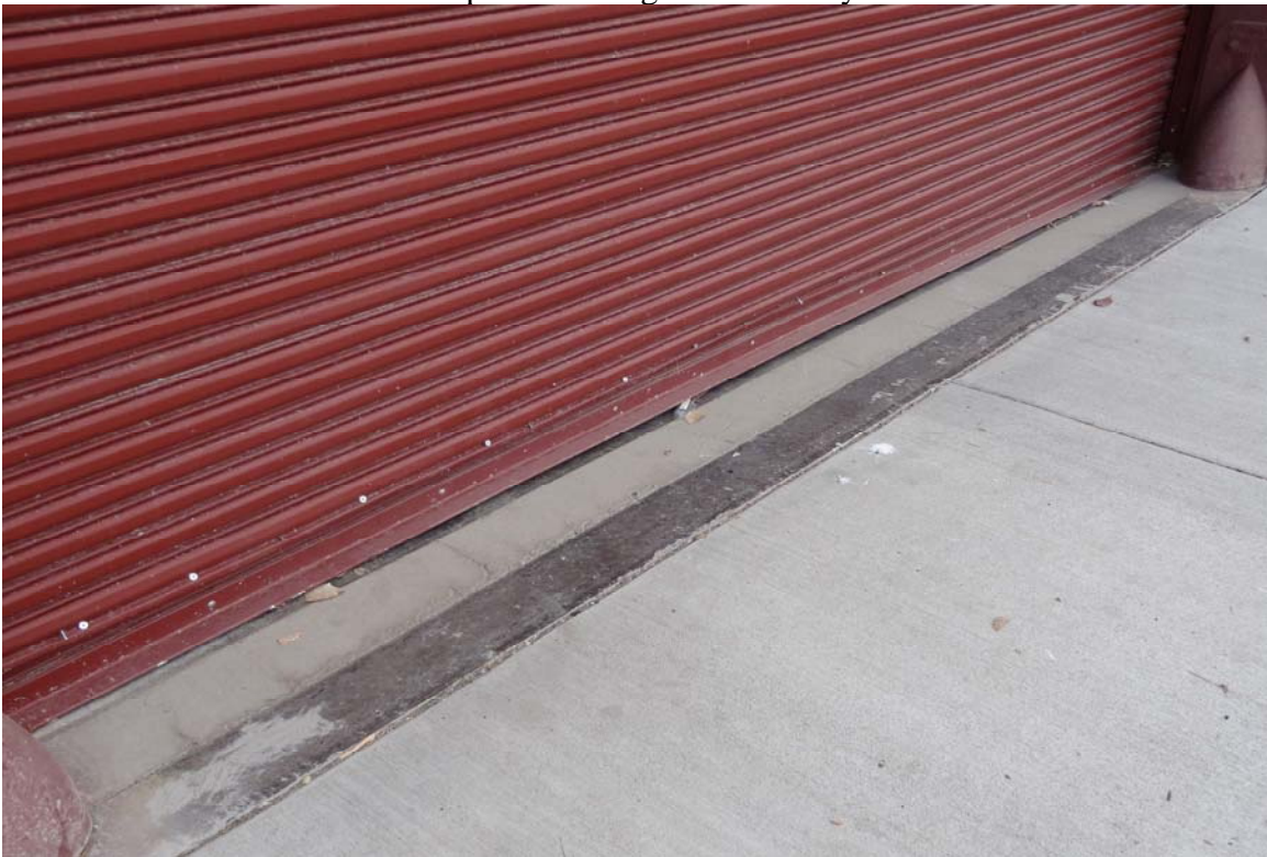
Fallon Armory - Building #0678 Description: Damaged overhead coiling door.
