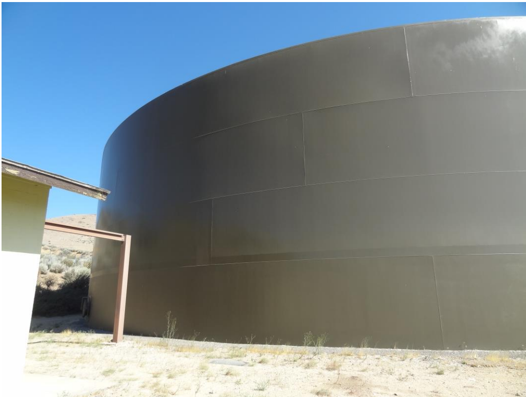
Marlette Lake 1 Million Gallon Tank - Building #2486 Description: Exterior finishes needed.
