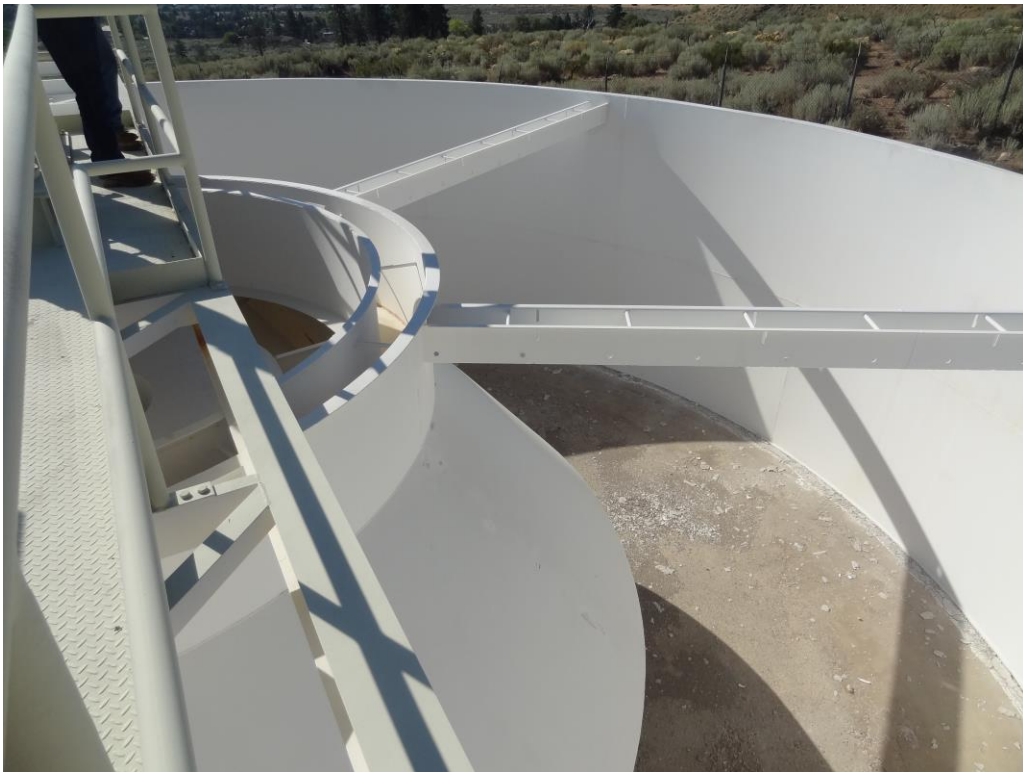
Marlette 1.5 Gallon Storage Tank - Building #2504 Description: Concrete foundation needed.
