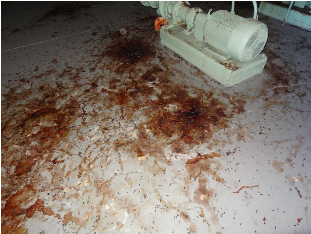
Marlette Lake Chlorine - Building #2489 Description: Pest control needed.
