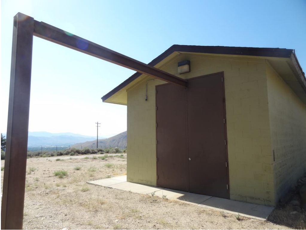
Marlette Lake Water Treatment - Building #2487 Description: Exterior finishes needed.
