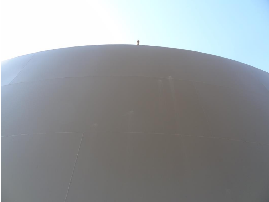
Marlette Lake 3 Million Gallon Tank - Building #2485 Description: Guardrails needed.
