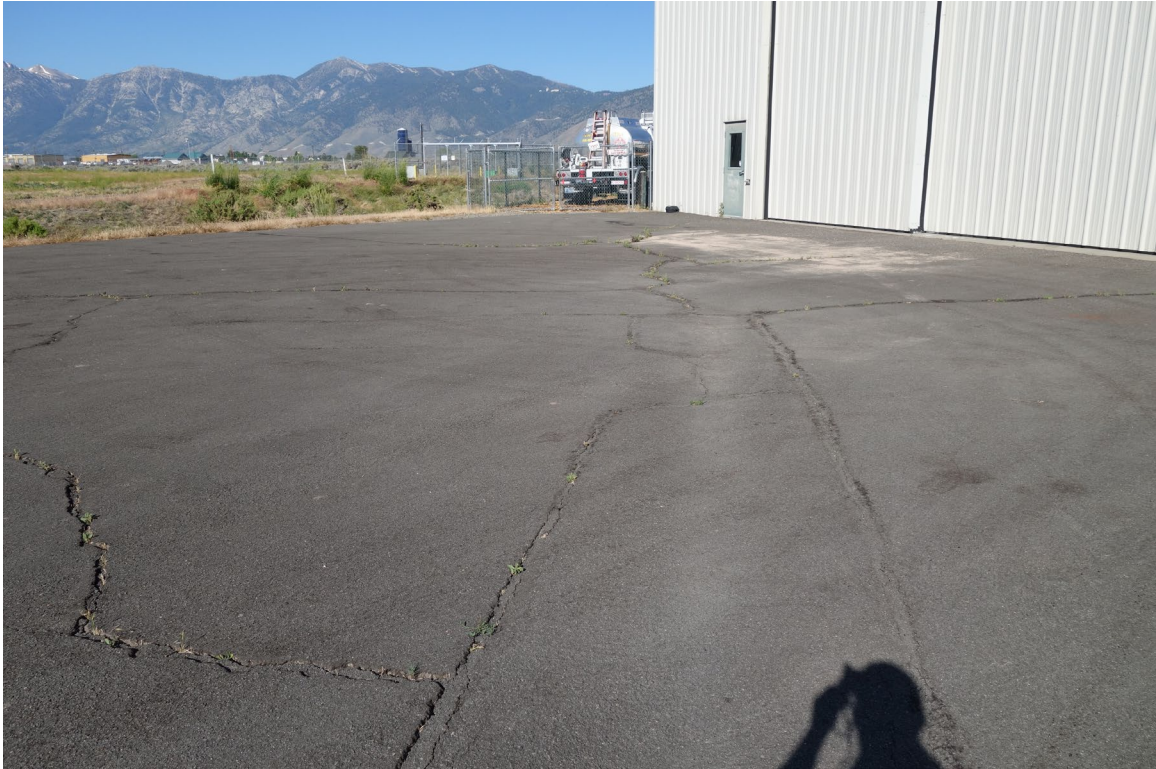
Sierra Front Interagency Dispatch Center Site – FCA Site #9900 Description: Regrade NDOW Hangar Apron.
