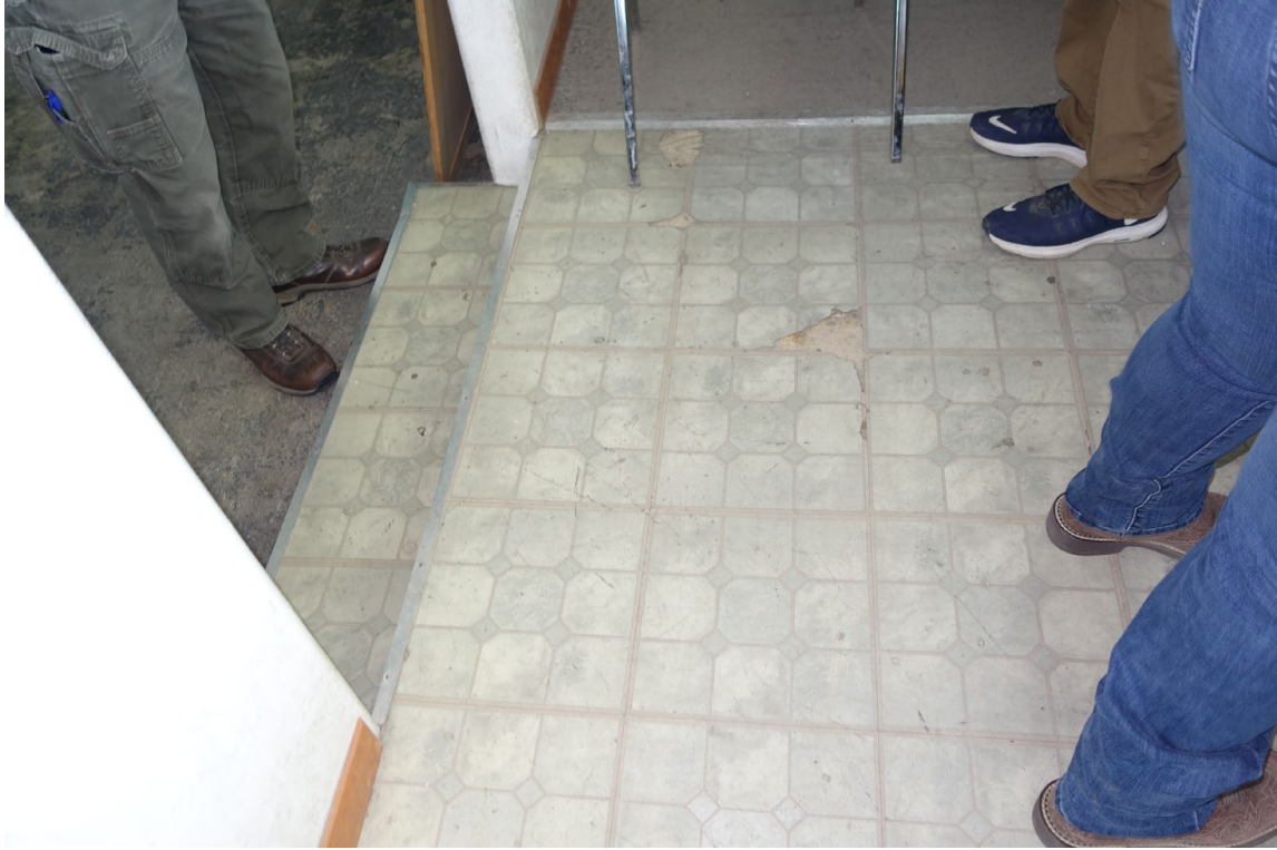
Sierra Front Interagency Hangar – FCA Building #2491 Description: Flooring Replacement Needed.
