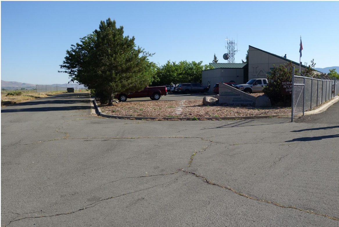
Sierra Front Interagency Dispatch Center – FCA Building #2490 Description: Exterior of the Building.
