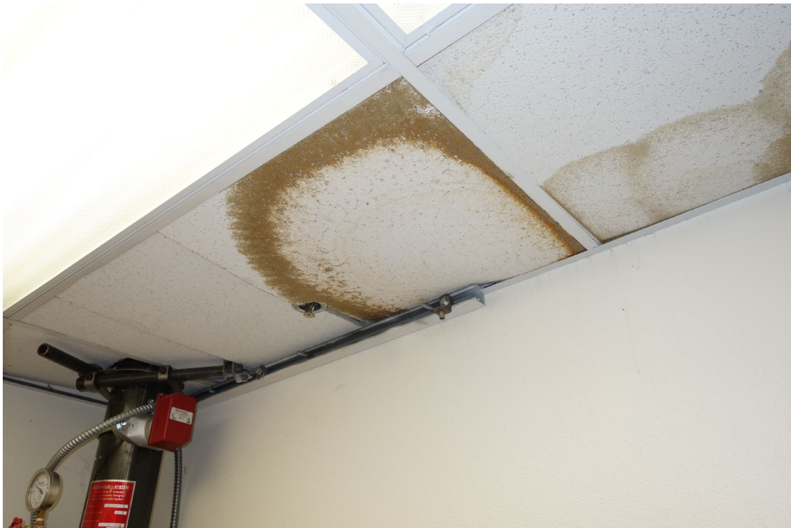
NDOW Aircraft Hangar – FCA Building #0661 Description: Leak Repairs Needed.
