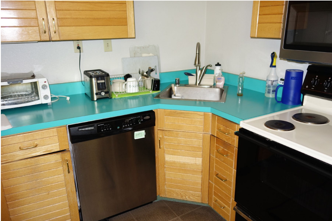
Sierra Front Interagency Dispatch Center – FCA Building #2490 Description: Non-Accessible Break Room Remodel Needed.
