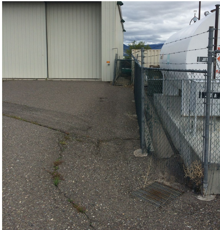
Sierra Front Interagency Dispatch Center Site – FCA Site #9900 Description: Fuel Tanks Containment & Drain Relocation Recommended.
