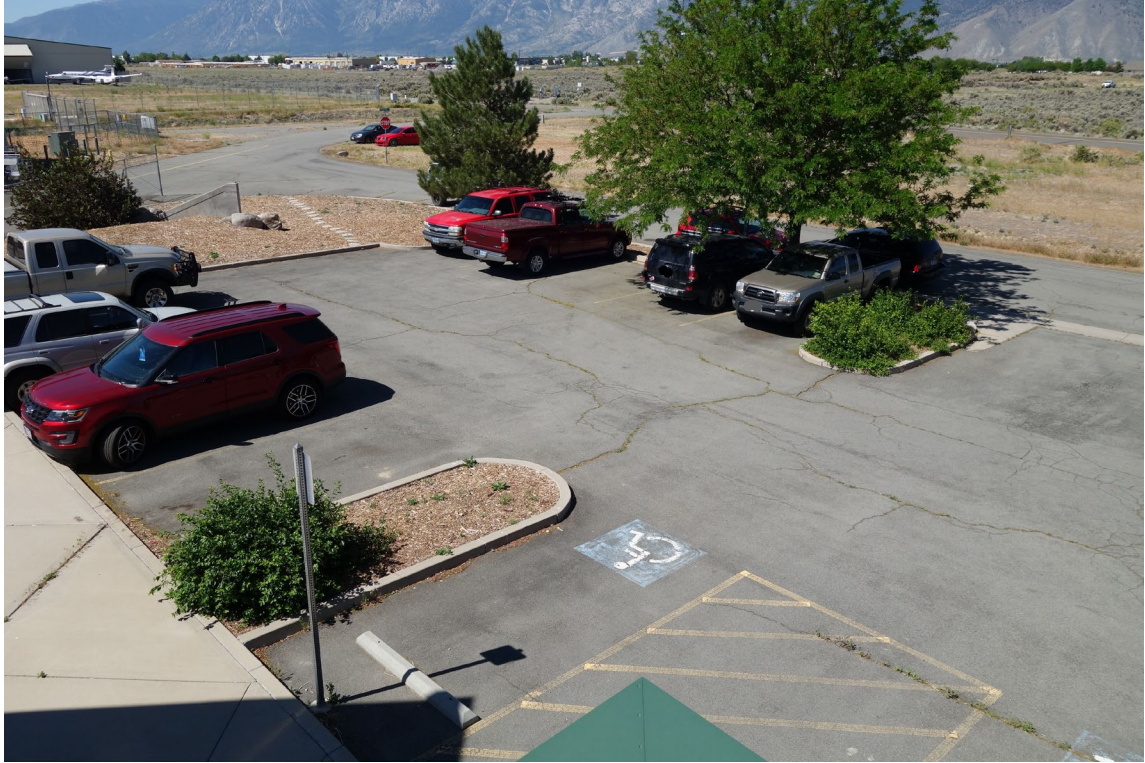
Sierra Front Interagency Dispatch Center Site – FCA Site #9900 Description: Crack Fill & Slurry Seal Needed.
