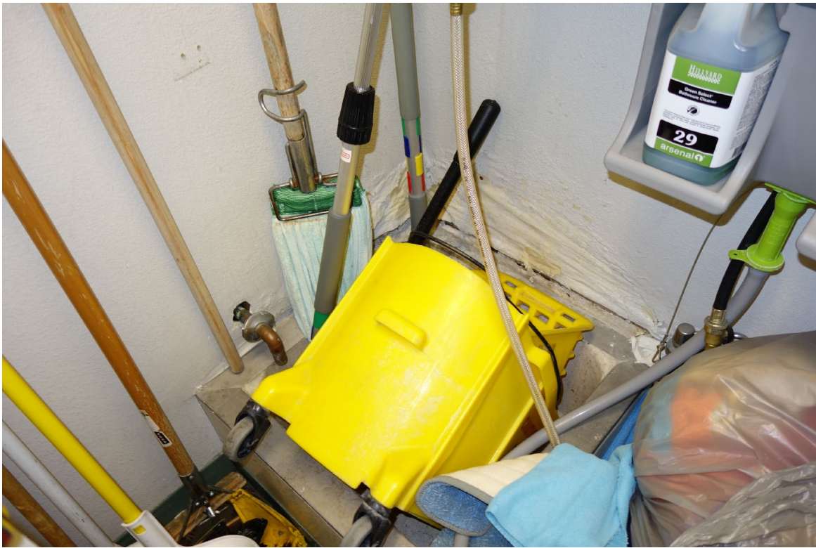
Sierra Front Interagency Dispatch Center – FCA Building #2490 Description: Janitors Closet Wall Repairs Needed.
