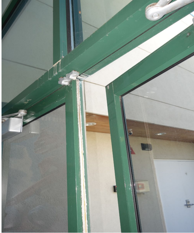
Sierra Front Interagency Dispatch Center – FCA Building #2490 Description: Storefront Door System Replacement Needed.
