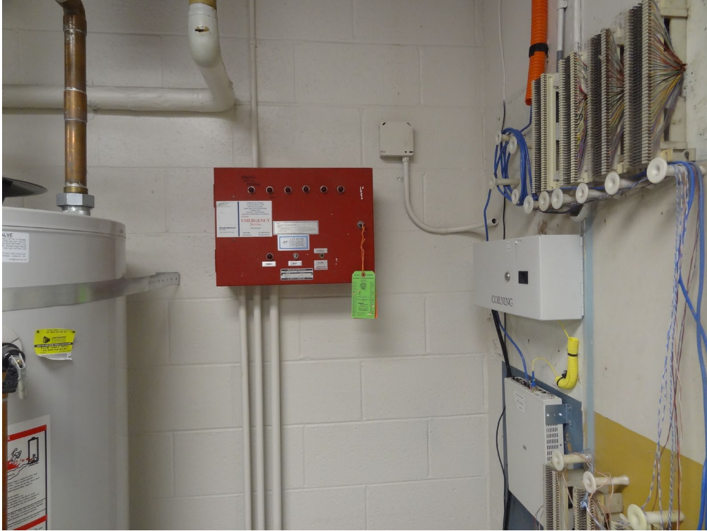
Henderson Armory - Building #0680 Description: Fire Alarm System Upgrades Needed.
