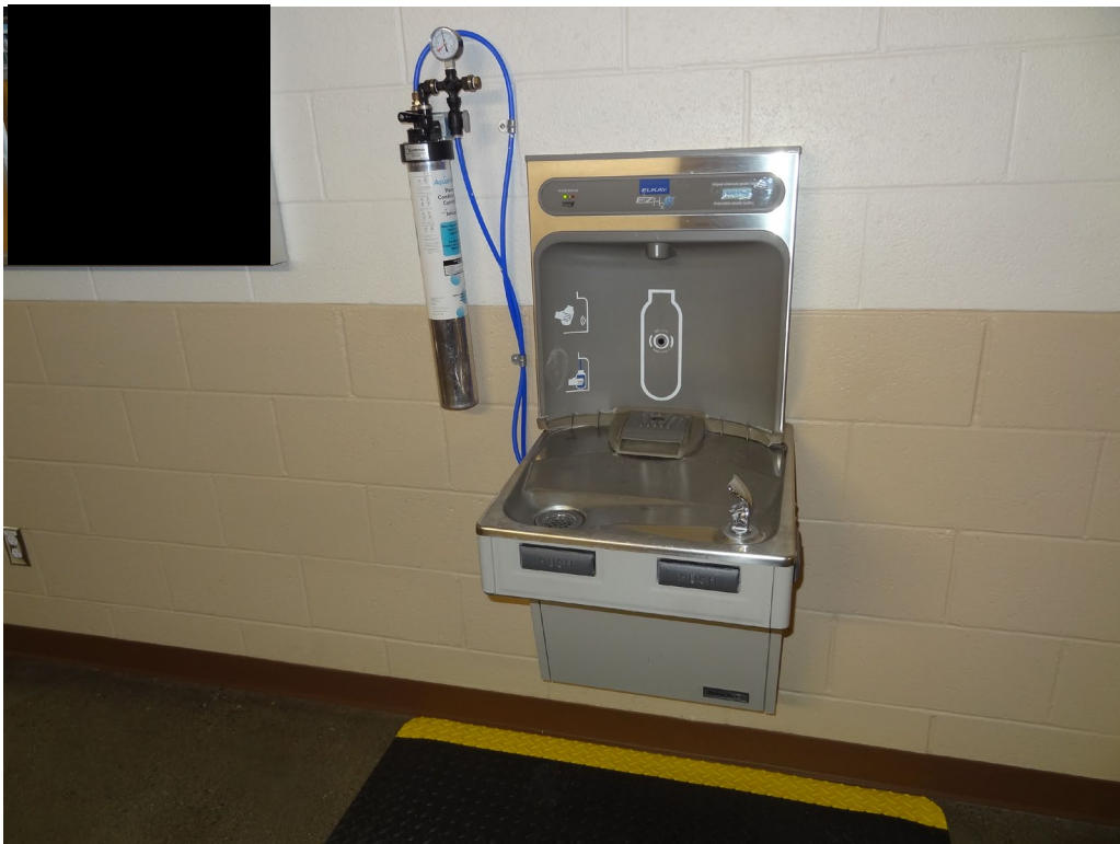
Henderson Armory - Building #0680 Description: Dual Level Drinking Fountain Installation Needed.
