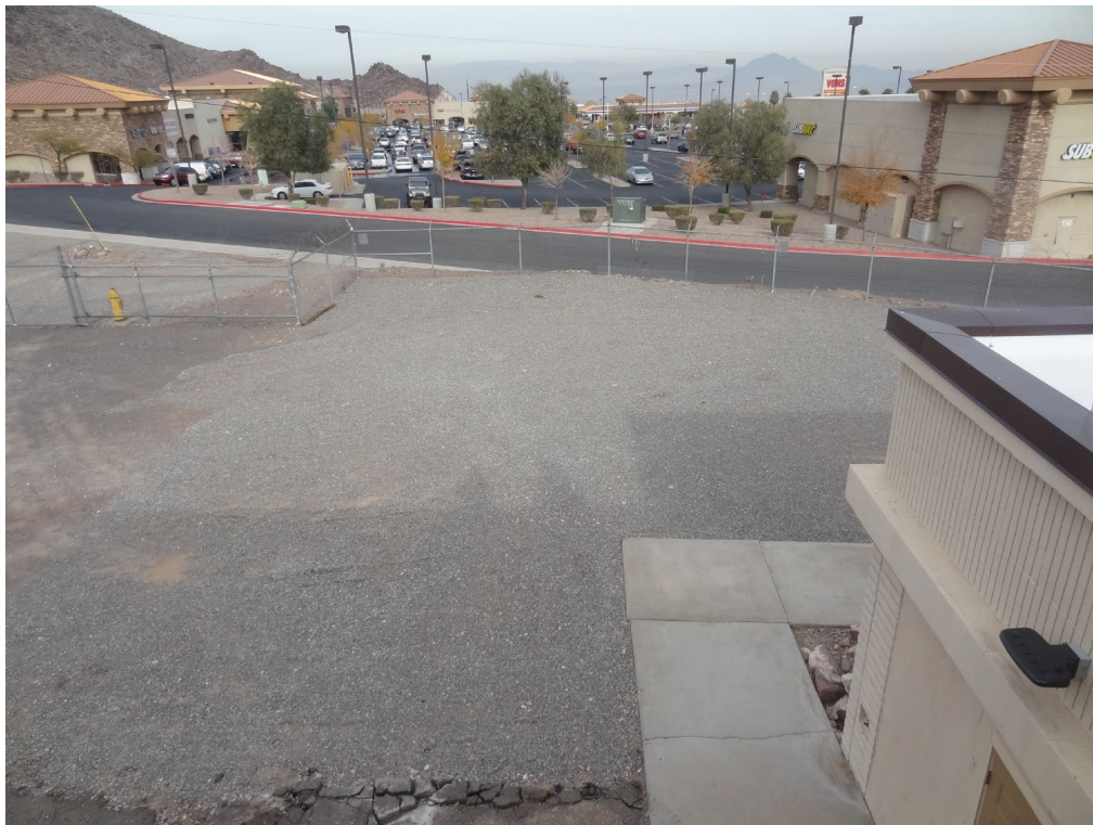
Henderson Armory - Site #9912 Description: Erosion Control Needed on North and South Sides.
