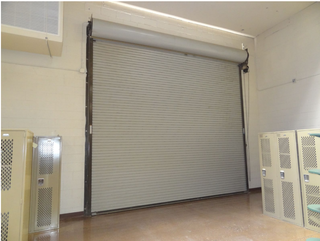
Henderson Armory - Building #0680 Description: Overhead Door Replacement Needed.
