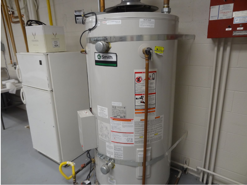
Henderson Armory - Building #0680 Description: Water Heater Replacement Needed.
