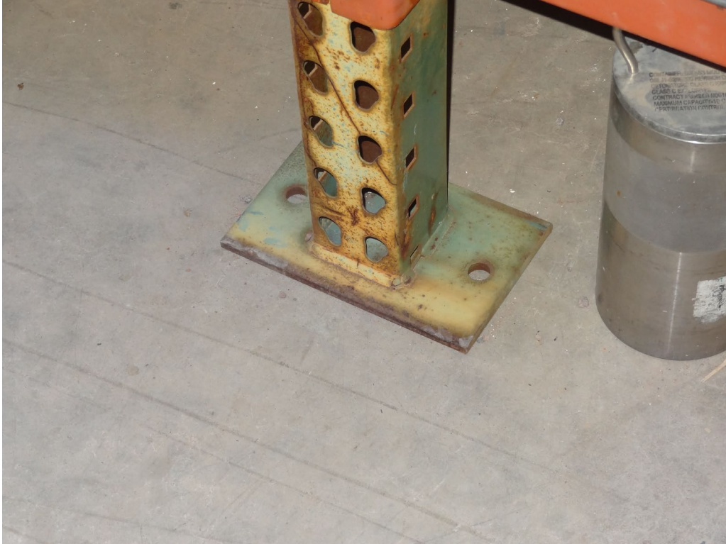
Henderson Armory Butler Building #1 South - Building #0682 Description: Shelves Missing Proper Anchoring.
