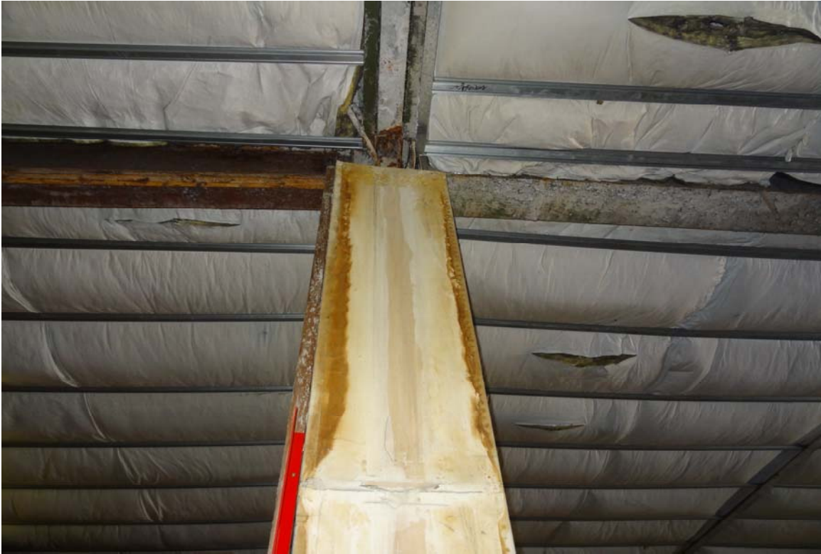
Las Vegas Purchasing Warehouse - Building #2395 Description: Water damage at columns.
