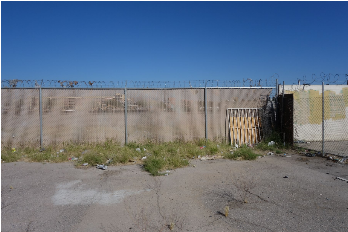
Las Vegas Purchasing Warehouse Site - Site #9914 Description: Weed and Debris Combustible Accumulation.
