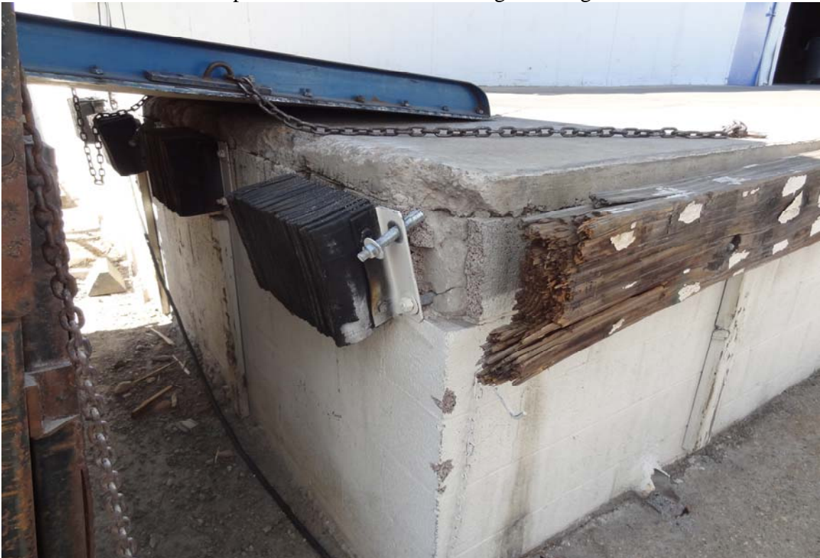
Las Vegas Purchasing Warehouse - Building #2395 Description: Damaged loading dock.
