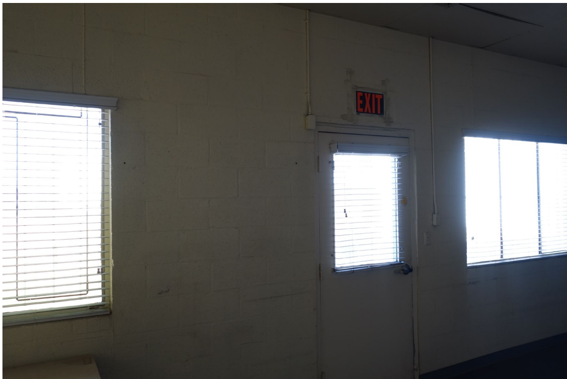
Las Vegas Purchasing Warehouse - Building #2395 Description: Exit Sign & Egress Lighting Needed.
