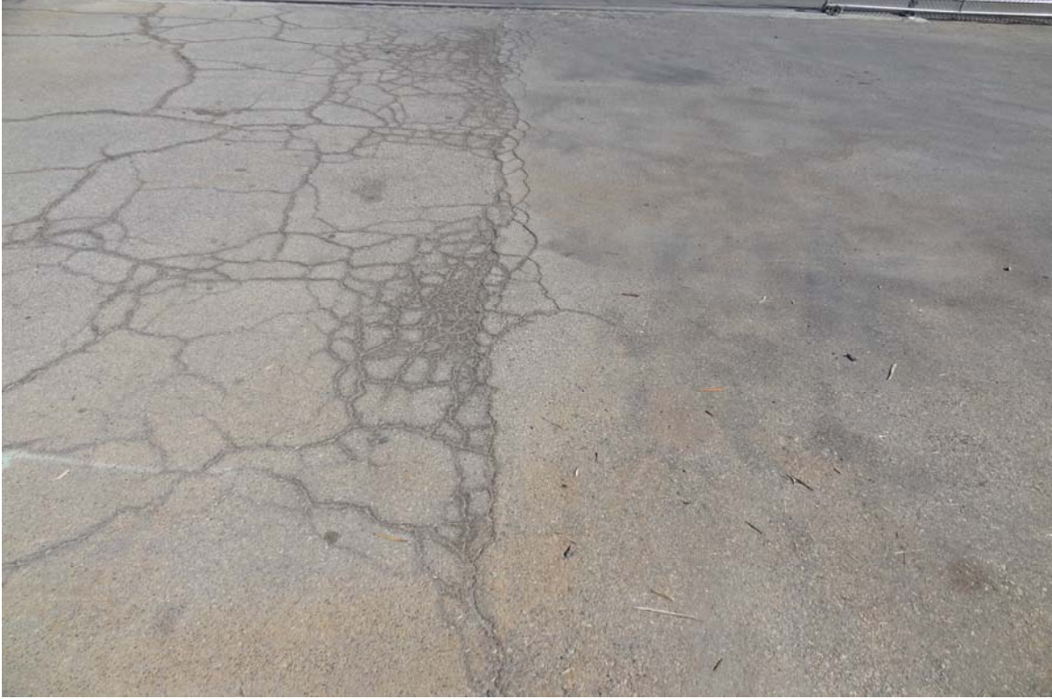
Las Vegas Purchasing Warehouse Site - Site #9914 Description: Damaged asphalt paving.
