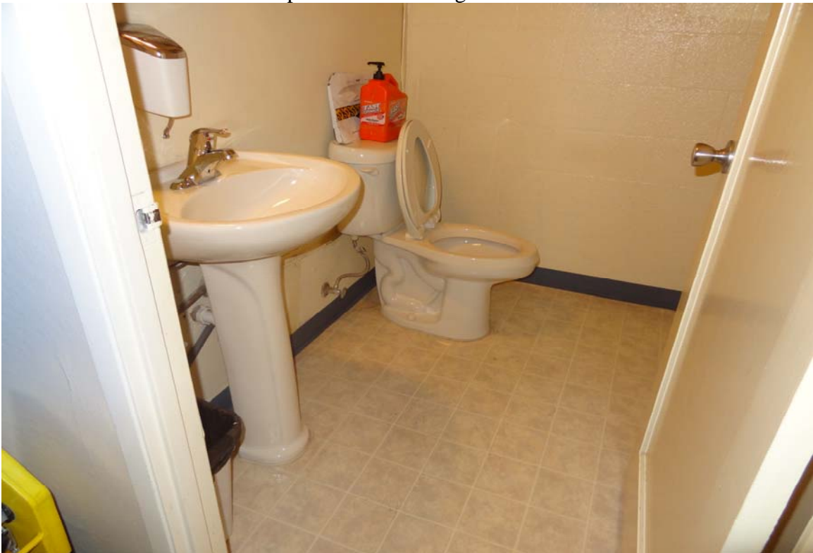
Las Vegas Purchasing Warehouse - Building #2395 Description: Non ADA compliant restroom.
