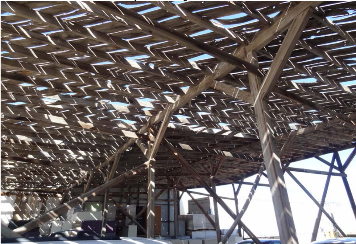
Purchasing Warehouse Carport - Building #2396 Description: Structural damage to carport.
