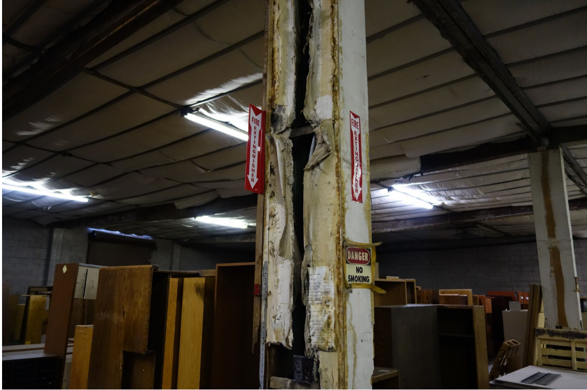
Las Vegas Purchasing Warehouse - Building #2395 Description: Missing Fire Extinguisher.
