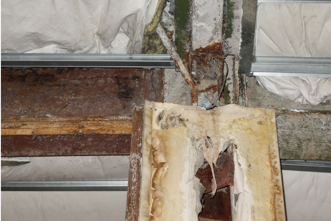
Las Vegas Purchasing Warehouse - Building #2395 Description: Column Repairs due to Water Damage.
