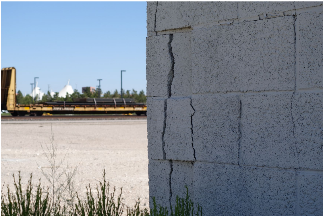
Las Vegas Purchasing Warehouse - Building #2395 Description: Damaged CMU Walls.
