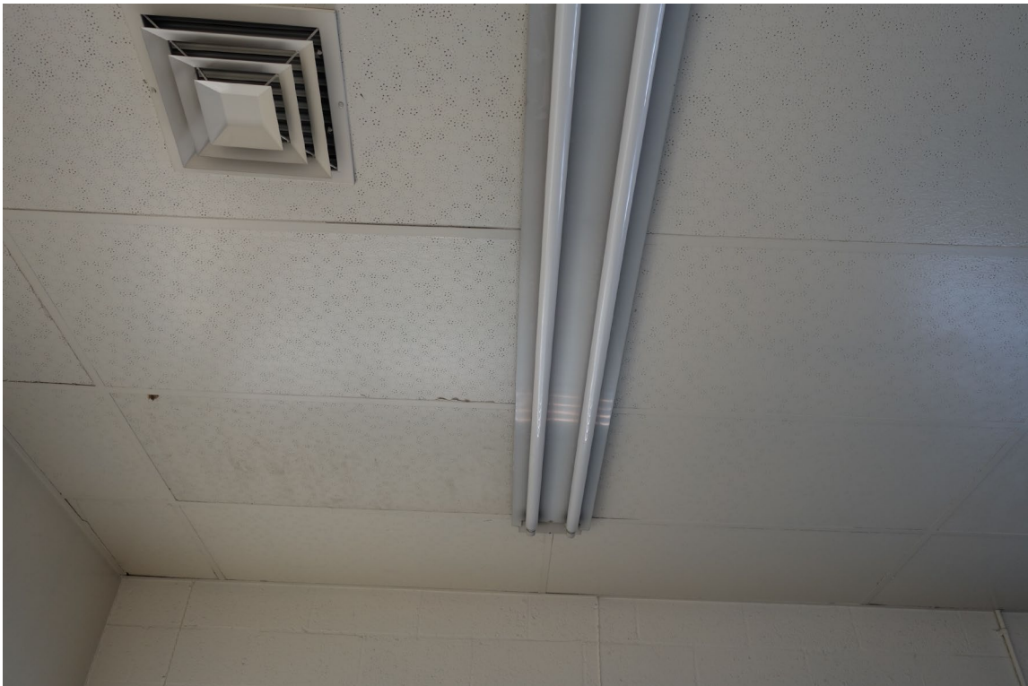
Las Vegas Purchasing Warehouse - Building #2395 Description: Lighting Upgrade Needed.
