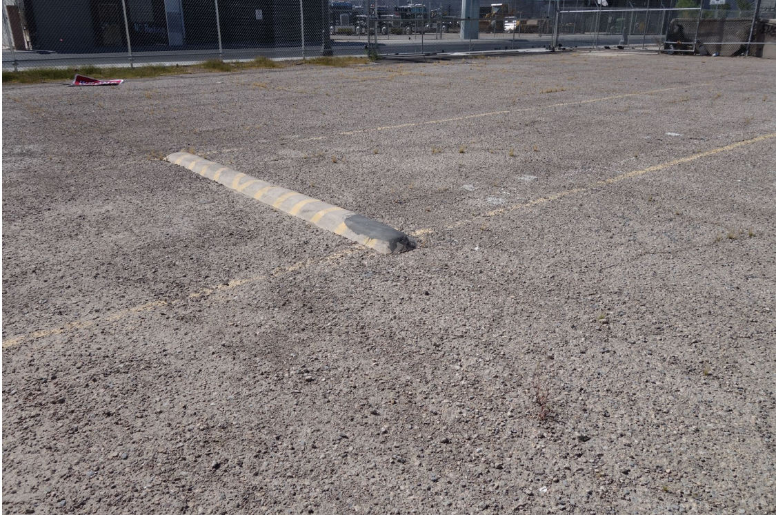
Las Vegas Purchasing Warehouse Site - Site #9914 Description: Asphalt Paving Replacement Needed.
