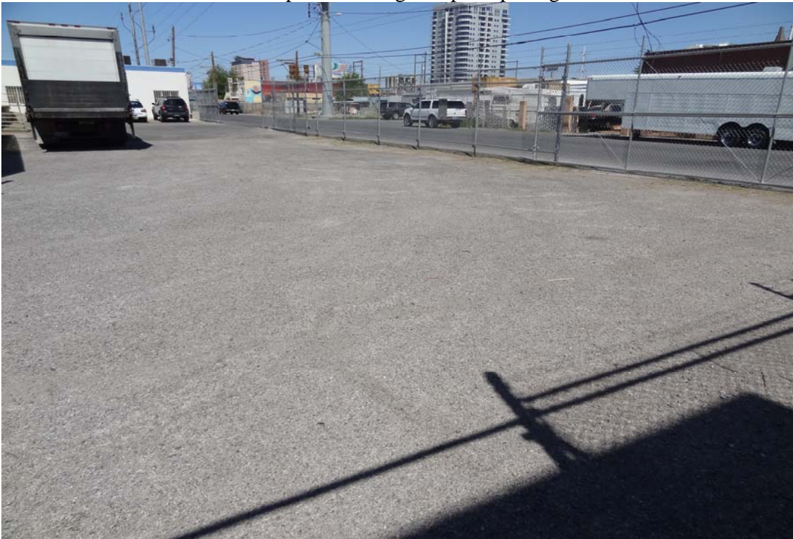
Las Vegas Purchasing Warehouse Site - Site #9914 Description: Damaged asphalt paving and fence.
