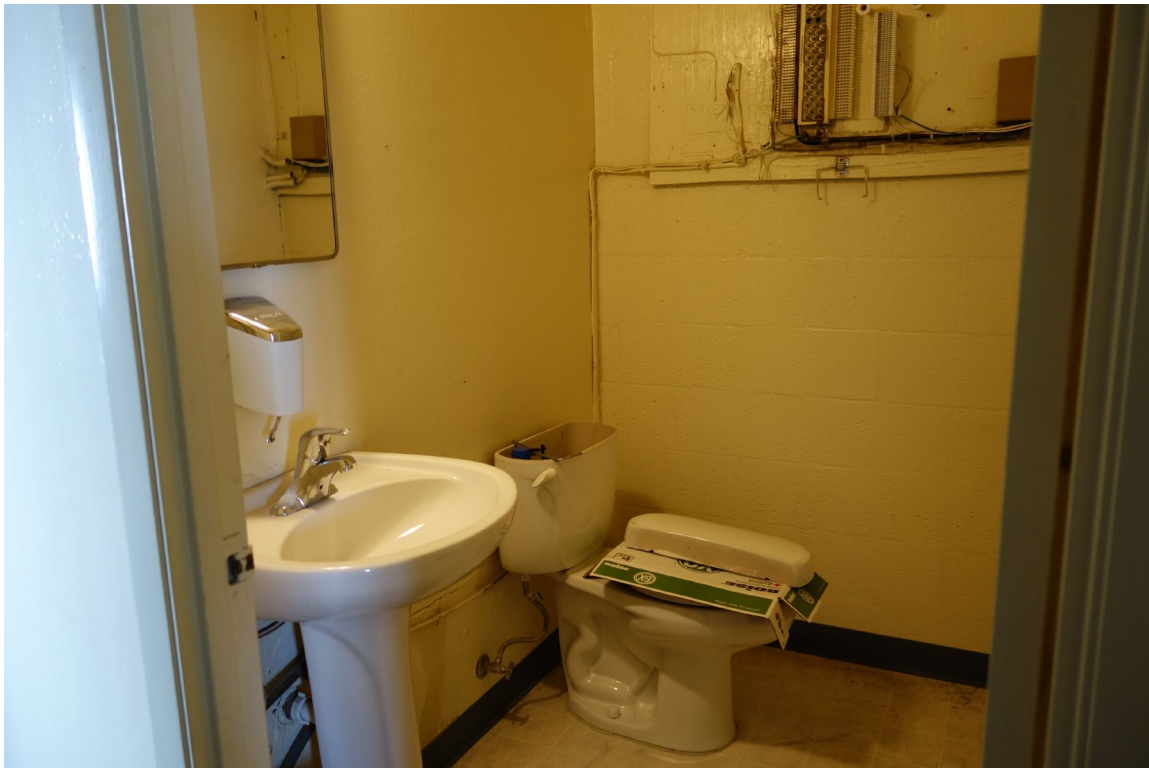
Las Vegas Purchasing Warehouse - Building #2395 Description: Restroom Remodel Needed.
