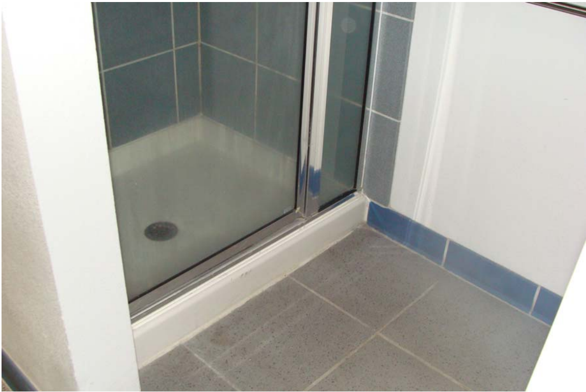
Reno NHP Headquarters - Building #0056 Description: Locker room shower in need of an ADA upgrade.
