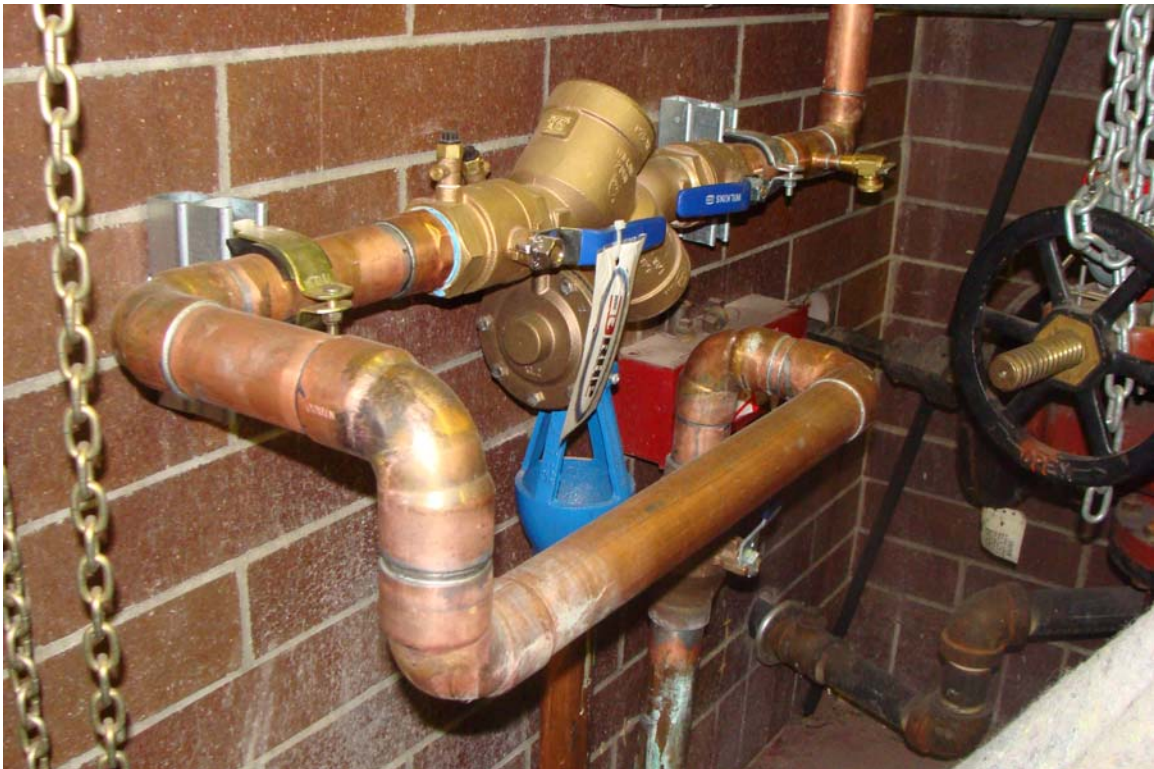
Regional Headquarters Shop / Garage - Building #1682 Description: View of domestic water check valve.
