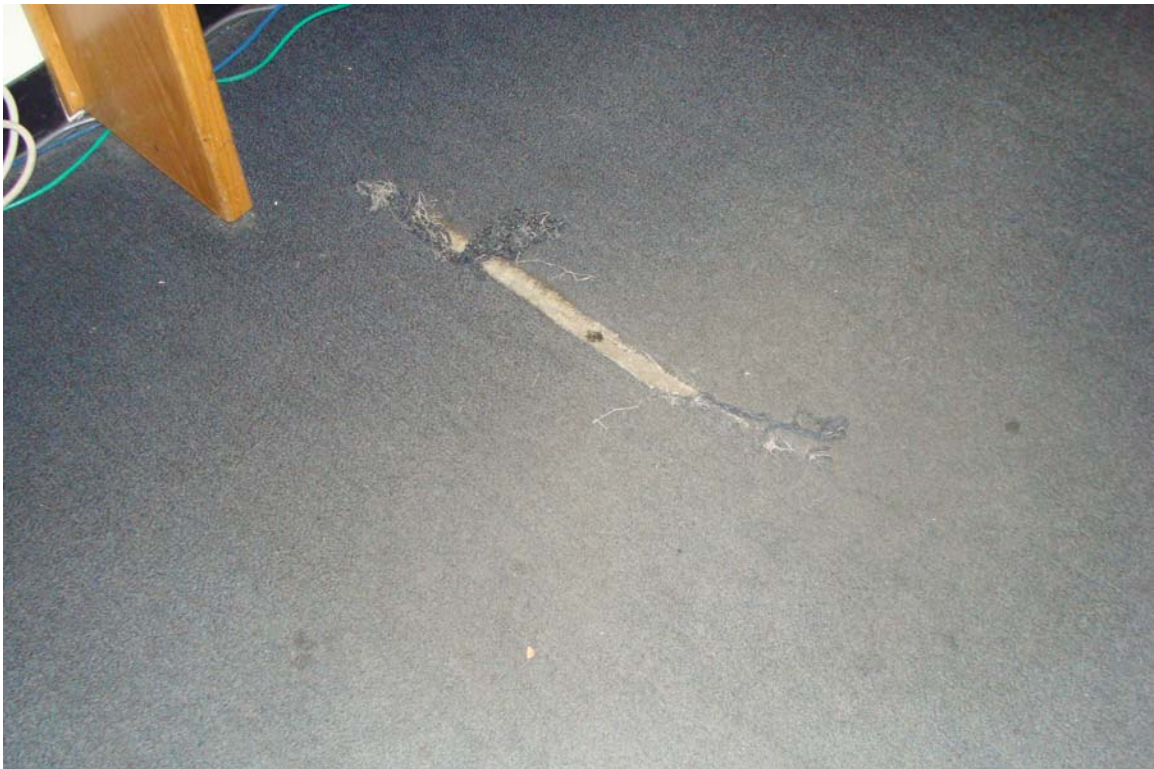
Reno NHP Headquarters - Building #0056 Description: Damaged carpet in report writing room.
