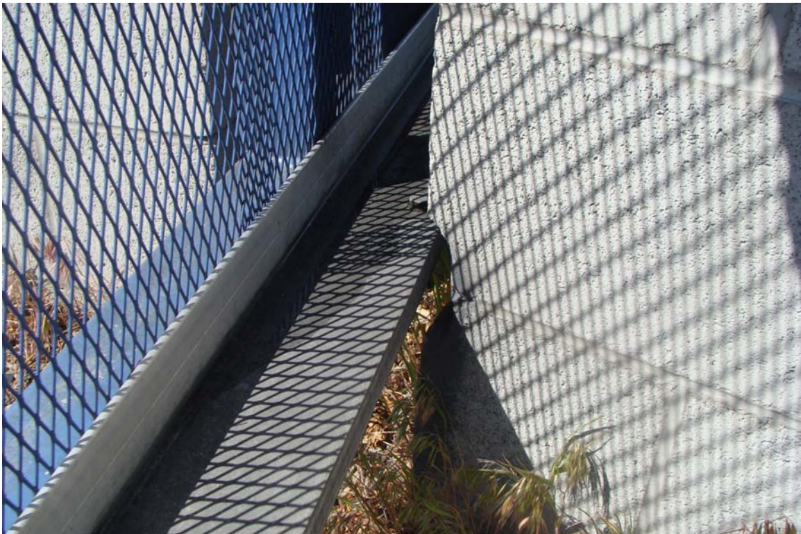
Reno NHP Headquarters Site - Site #9923 Description: Security gate rubbing on CMU wall.
