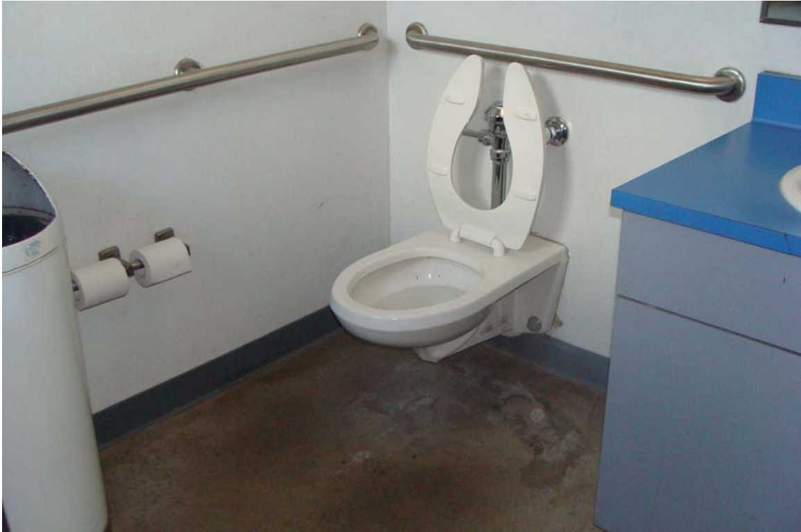
Regional Headquarters Shop / Garage - Building #1682 Description: View of the ADA restroom, note flush handle on wrong side.
