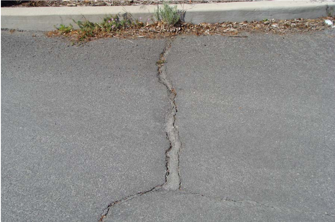
Reno NHP Headquarters Site - Site #9923 Description: AC paving in need of crack filling and sealing.
