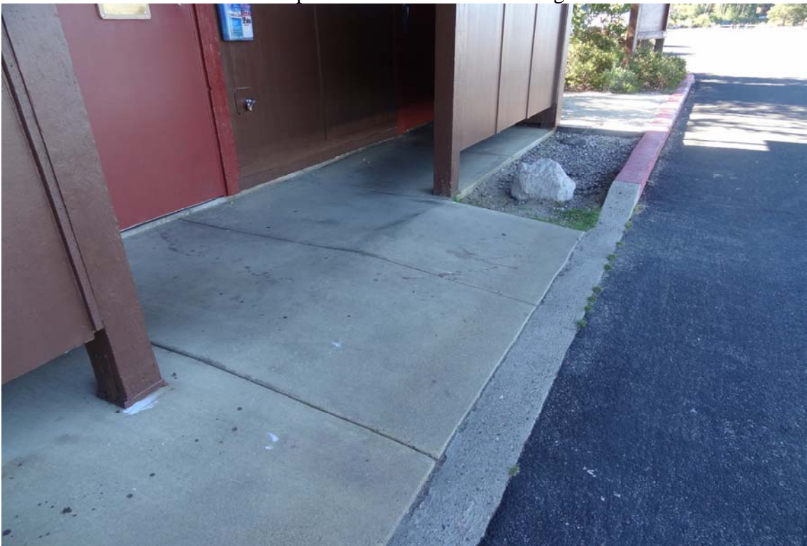
Cave Rock Comfort Station – FCA Building #0597 Description: Non-ADA compliant entrance.
