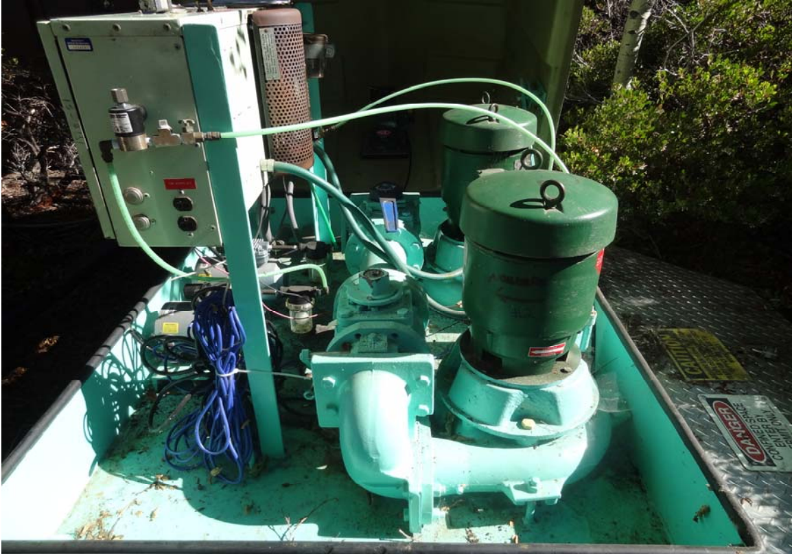
Cave Rock Sewer Pump Station – FCA Building #0583 Description: View of the pumps & equipment.
