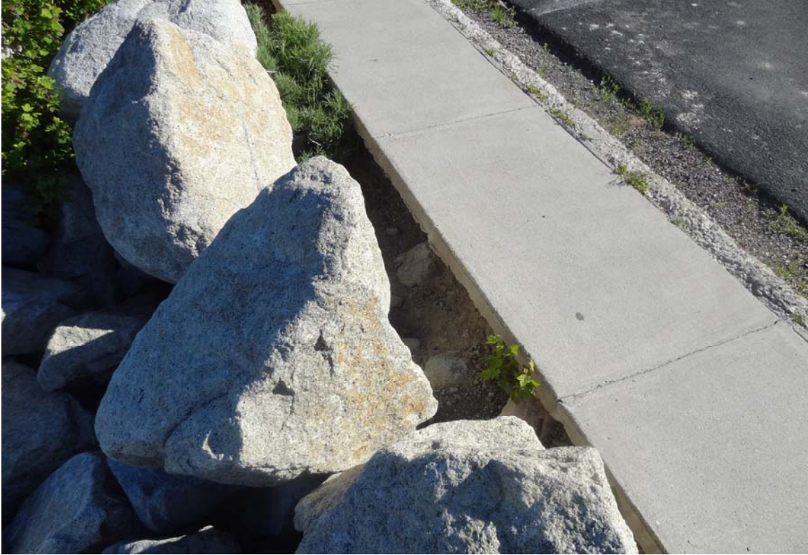
Lake Tahoe Nevada State Park – Cave Rock Site – FCA Site #9926 Description: Undermining of walkway due to erosion from wave action.
