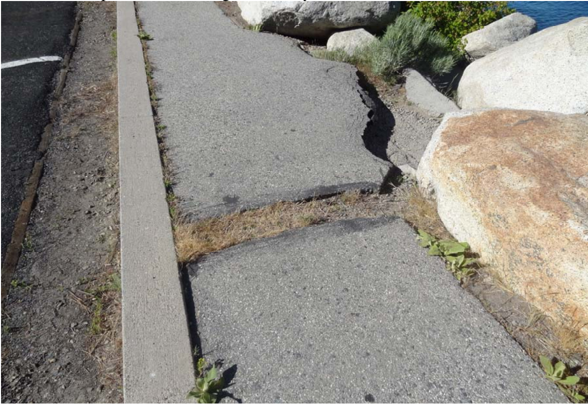
Lake Tahoe Nevada State Park – Cave Rock Site – FCA Site #9926 Description: Damaged walkway along parking area.
