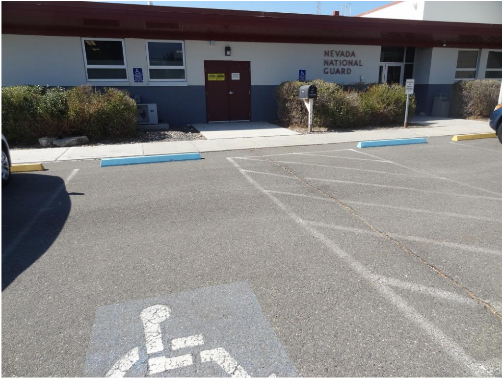
Elko Armory - Site #9937 Description: ADA parking stall striping needed.
