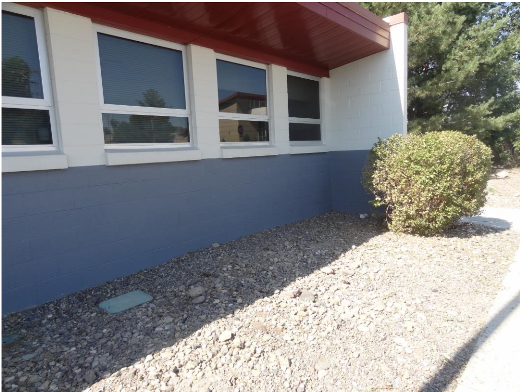
Armory – Building #0674 Description: Window replacement needed.
