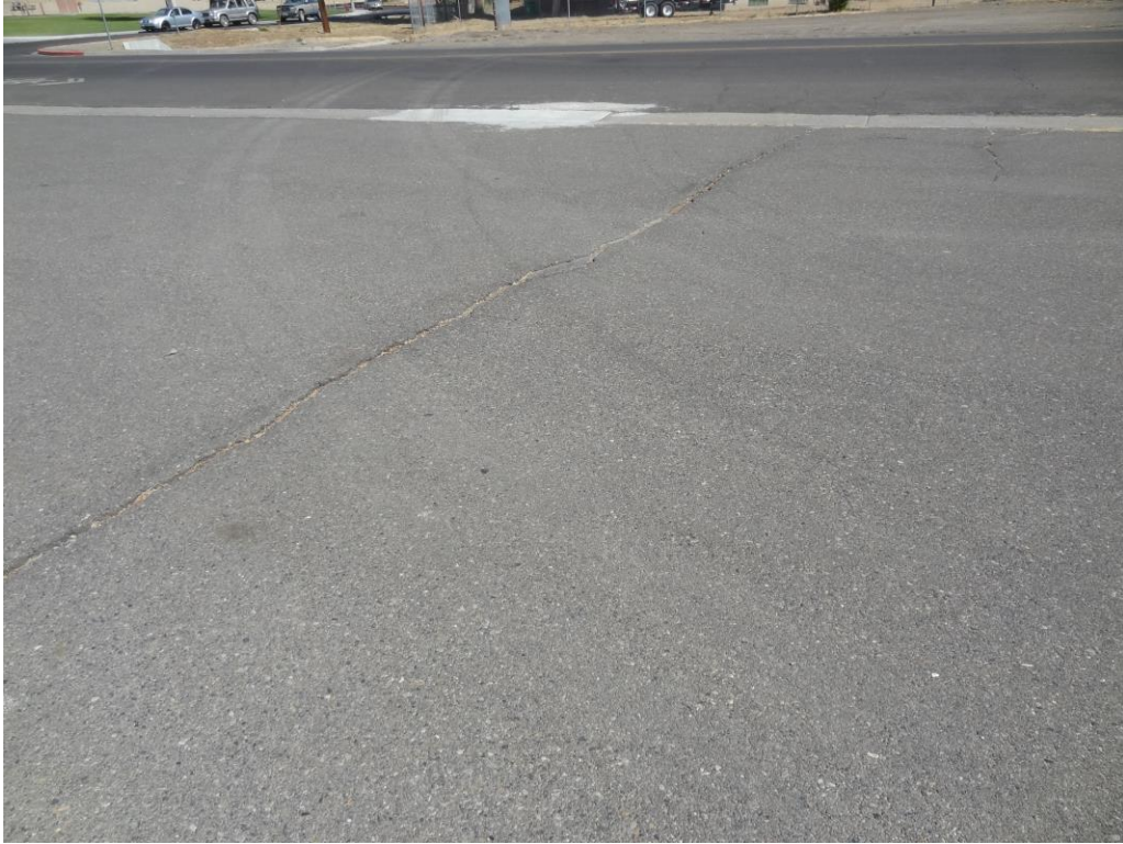
Elko Armory - Site #9937 Description: Slurry seal asphalt paving needed.
