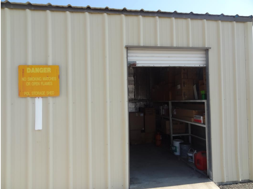
Hazardous Waste Storage #1 - Building #0677 Description: Safety Cabinets needed.
