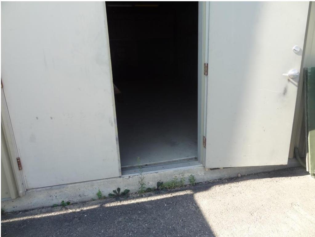
Storage Building - Building #1490 Description: Exterior landing installation needed.
