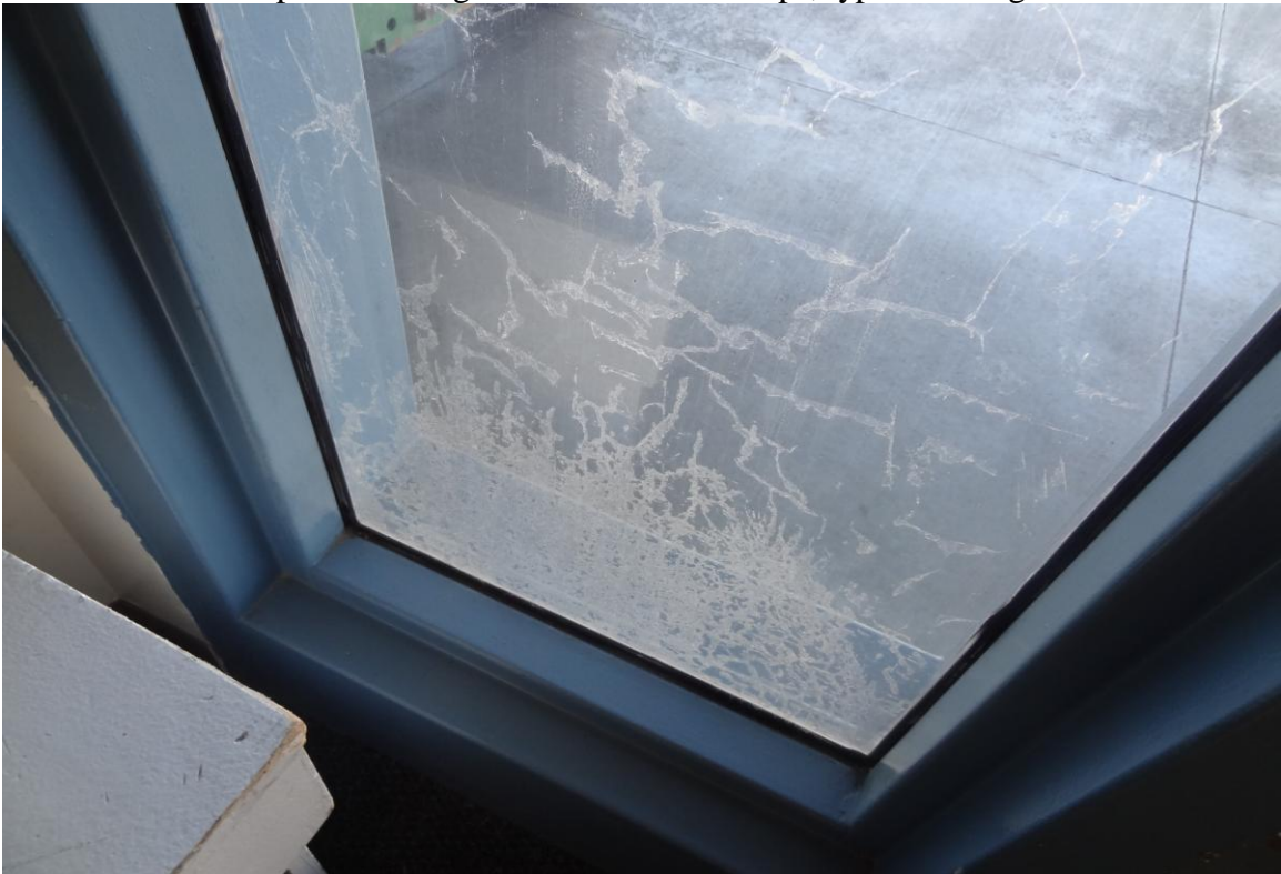
Building #9 Scheduled Services – FCA Building #1423 Description: Damaged glazing panel.
