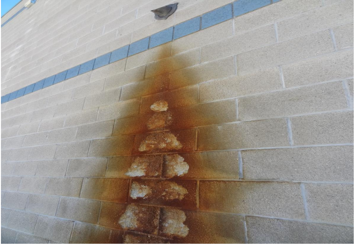
Building #11 Warehouse / Central Plant – FCA Building #1425 Description: Water damage to the exterior of the building.
