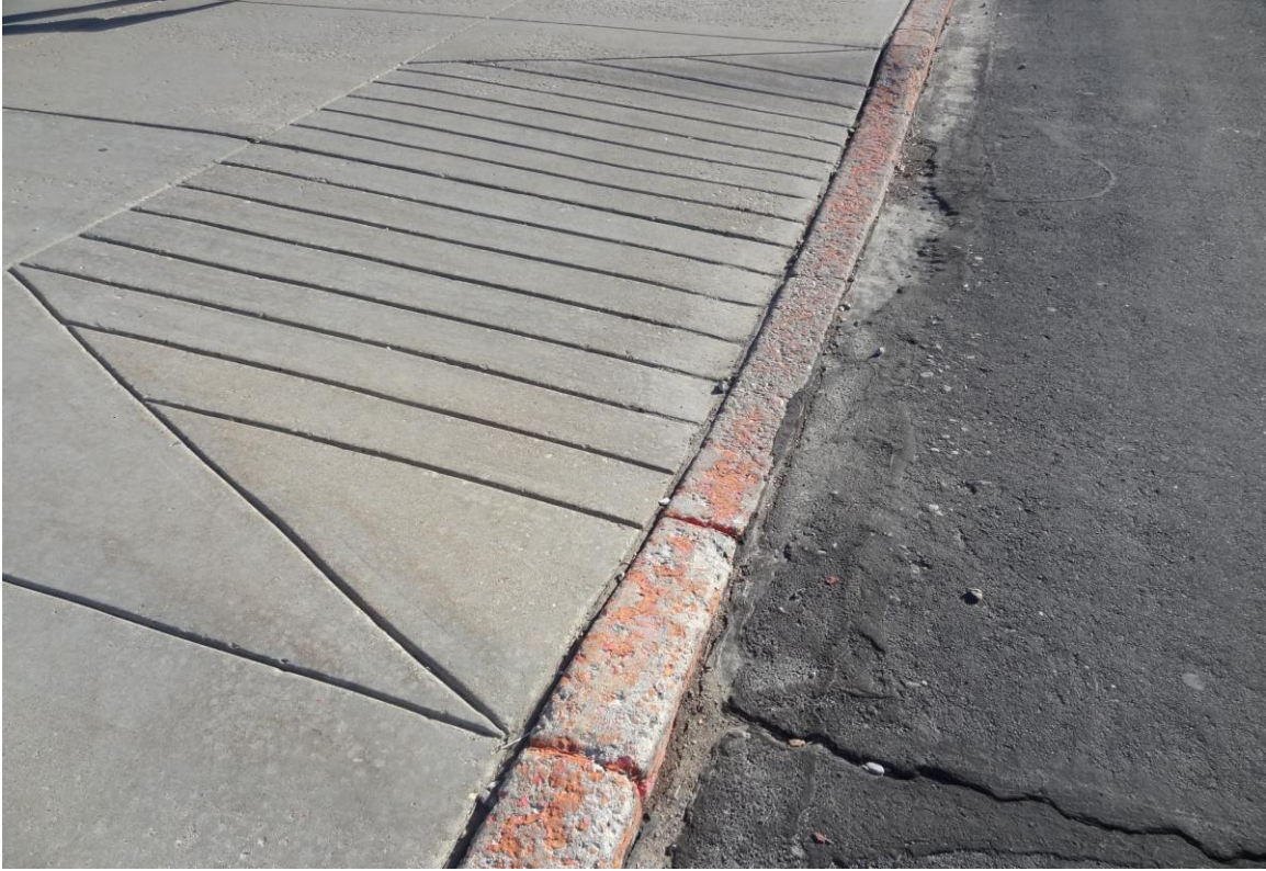
Ely State Prison Site – FCA Site #9941 Description: ADA accessible curb cut / paving damage.
