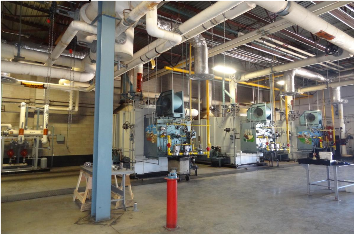
Building #11 Warehouse / Central Plant – FCA Building #1425 Description: Interior of the central plant.
