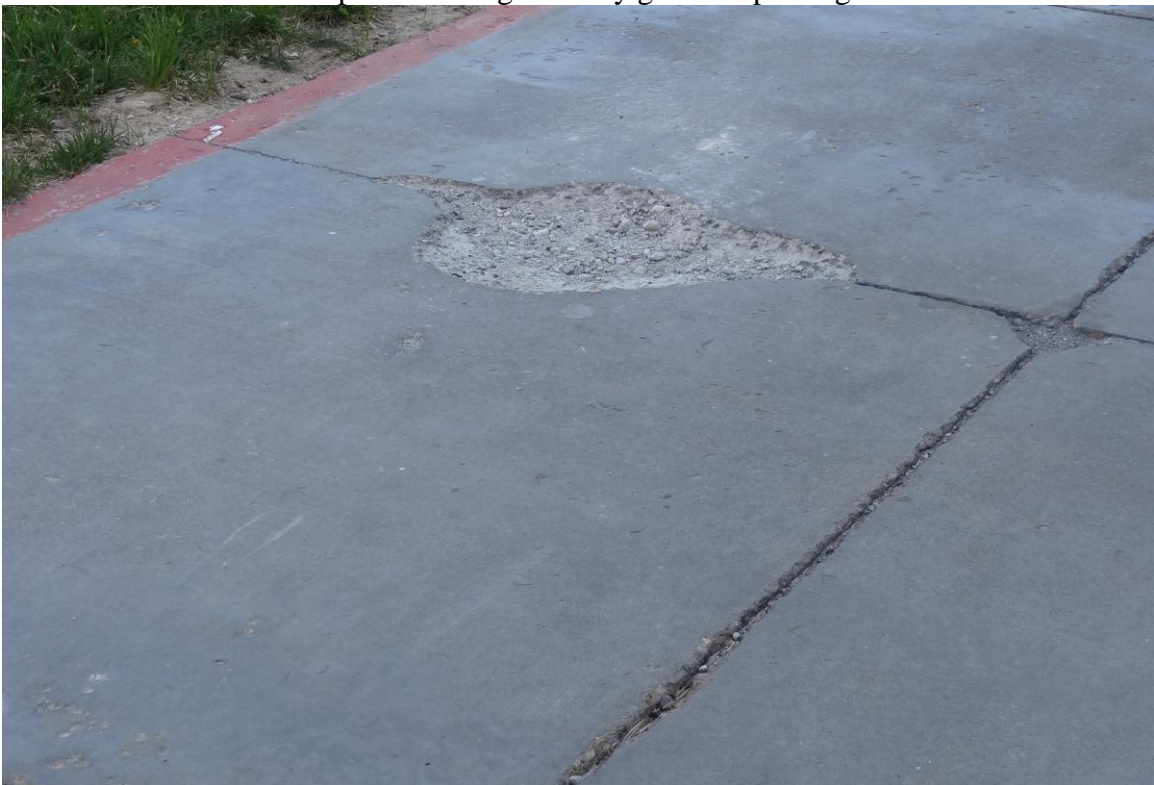
Ely State Prison Site – FCA Site #9941 Description: Damaged concrete walkway.
