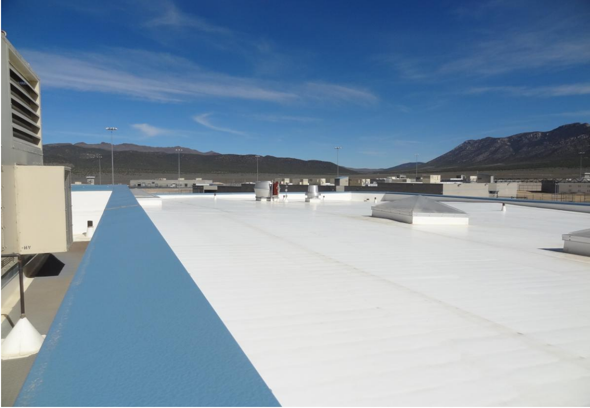
Housing Unit #8 – FCA Building #1422 Description: Roof of HU #8, typical of all housing units.
