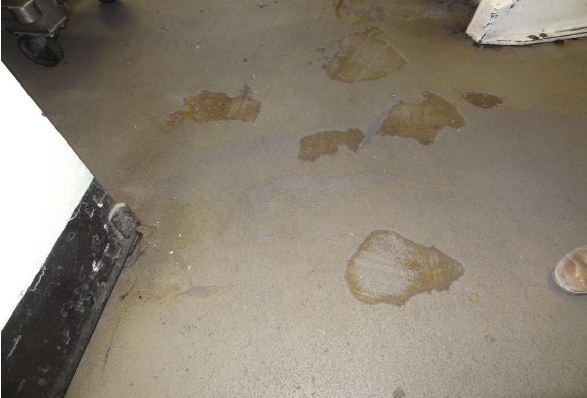
Building #10 Work & Recreation – FCA Building #1424 Description: Culinary floor damage.
