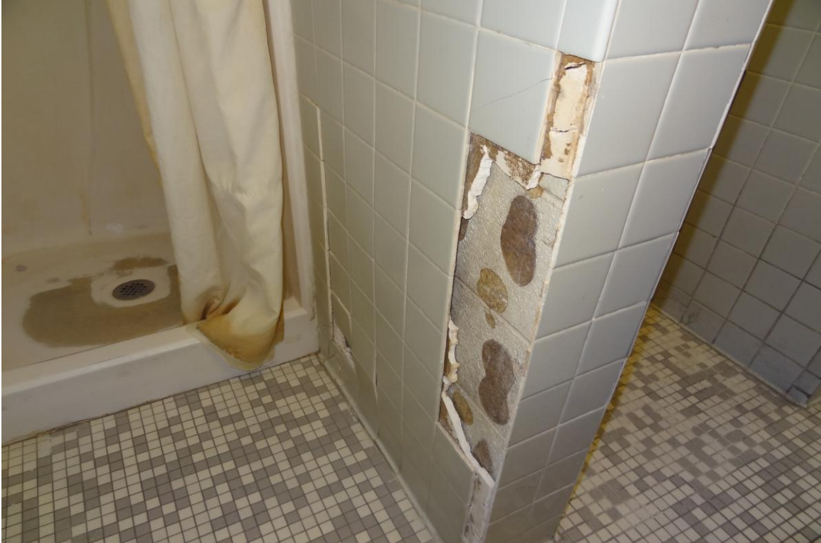
Building #12 Trustee Dormitory – FCA Building #1426 Description: Damaged tile in shower area.
