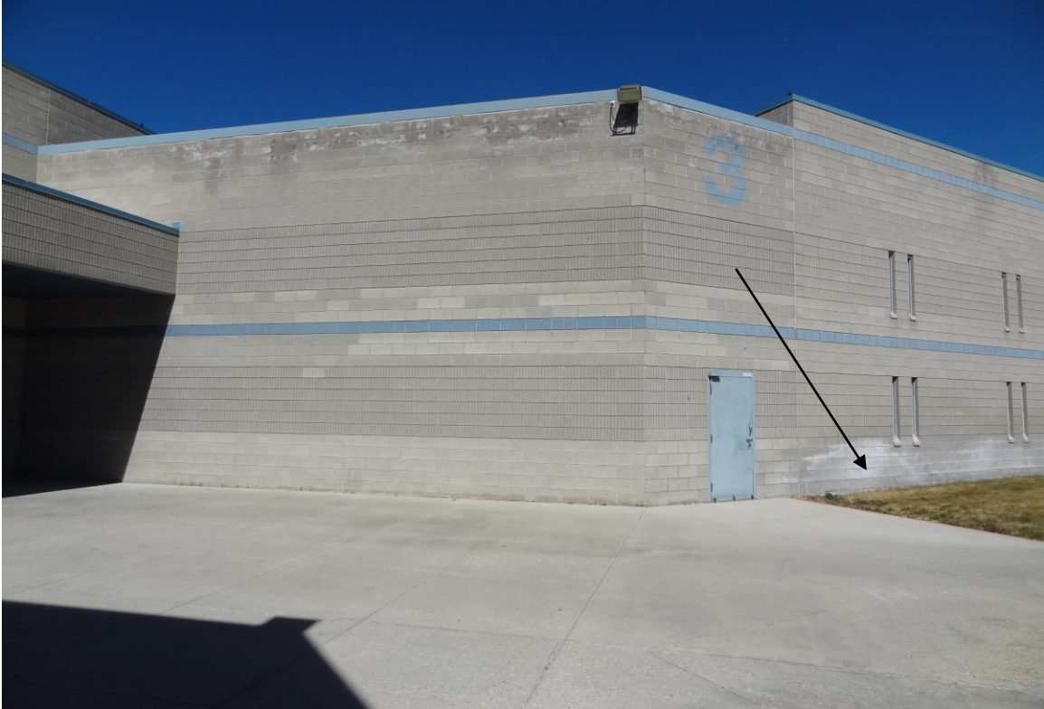
Housing Unit #3 – FCA Building #1417 Description: Typical exterior of housing unit, note water damaged CMU.
