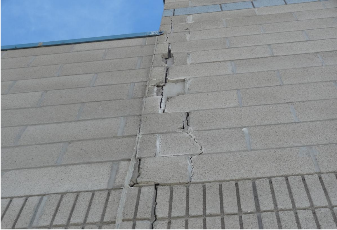
Building #10 Work & Recreation – FCA Building #1424 Description: Damaged CMU wall.
