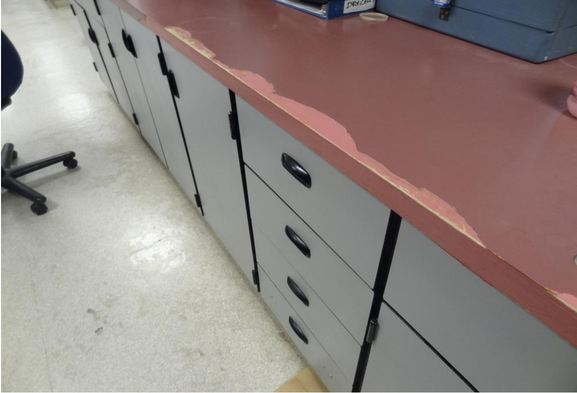
Building #9 Scheduled Services – FCA Building #1423 Description: Damaged laminate countertops, typical throughout.
