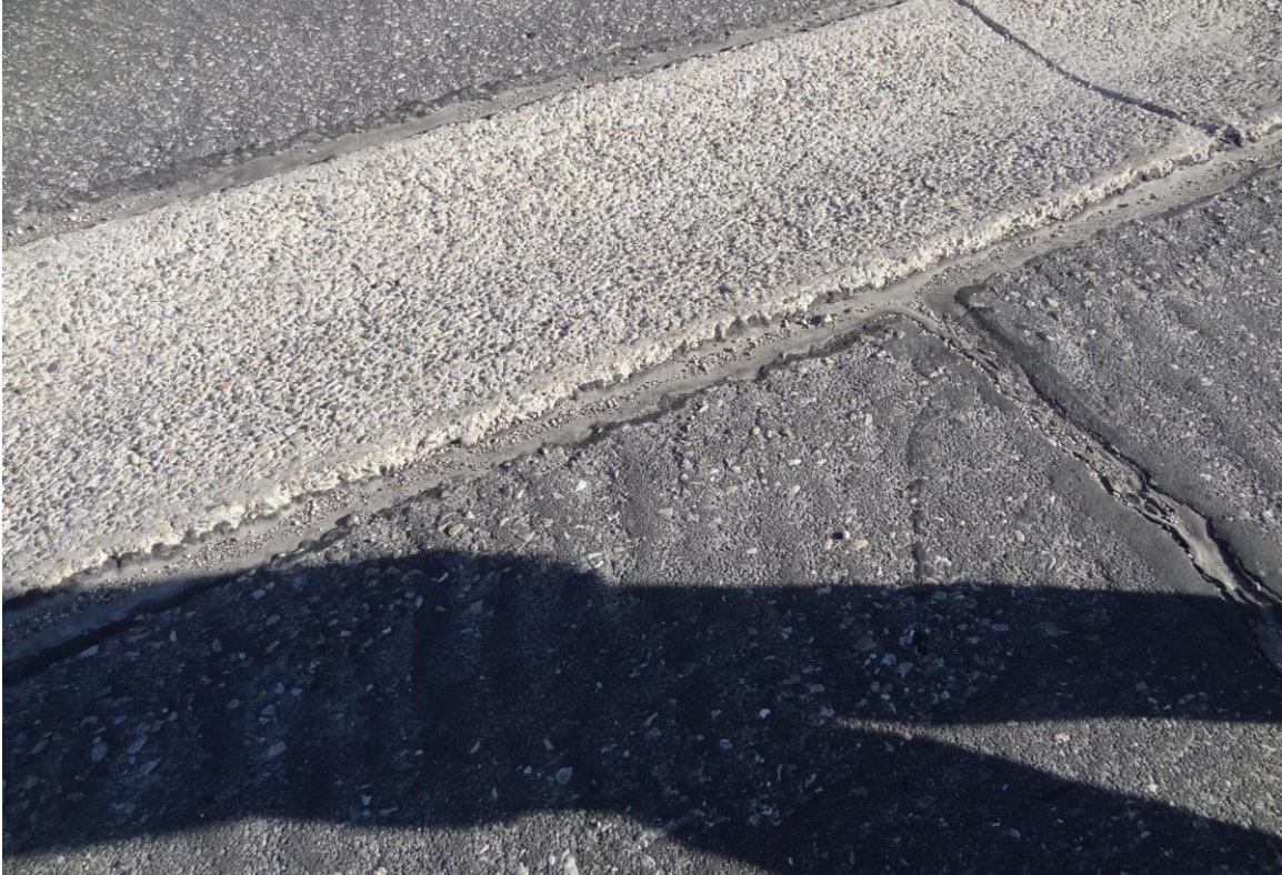
Ely State Prison Site – FCA Site #9941 Description: Damaged valley gutter in parking lot.
