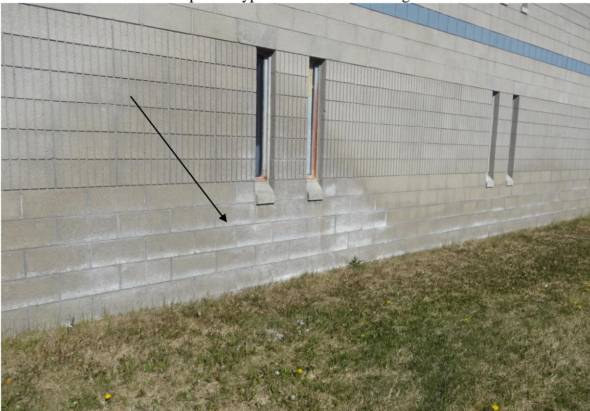
Housing Unit #7 – FCA Building #1421 Description: Typical exterior of housing unit, note water damaged CMU.
