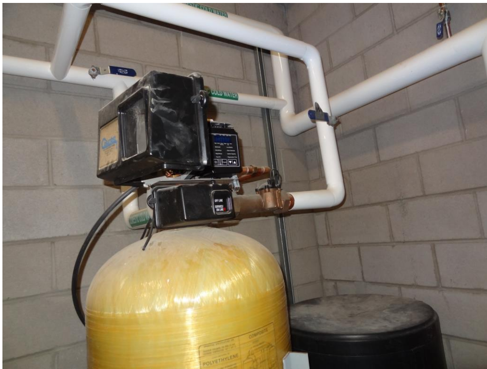
Visitation - Building #2093 Description: Water treatment system replacement needed.
