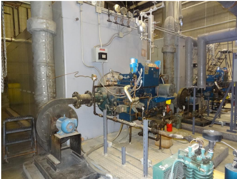
Maintenance/ Central Plant - Building #2097 Description: Boiler burner replacement needed.
