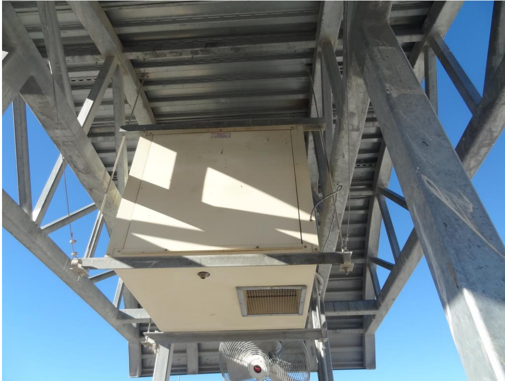
Housing Unit #8 - Building #2172 Description: Evaporative cooler replacement needed.
