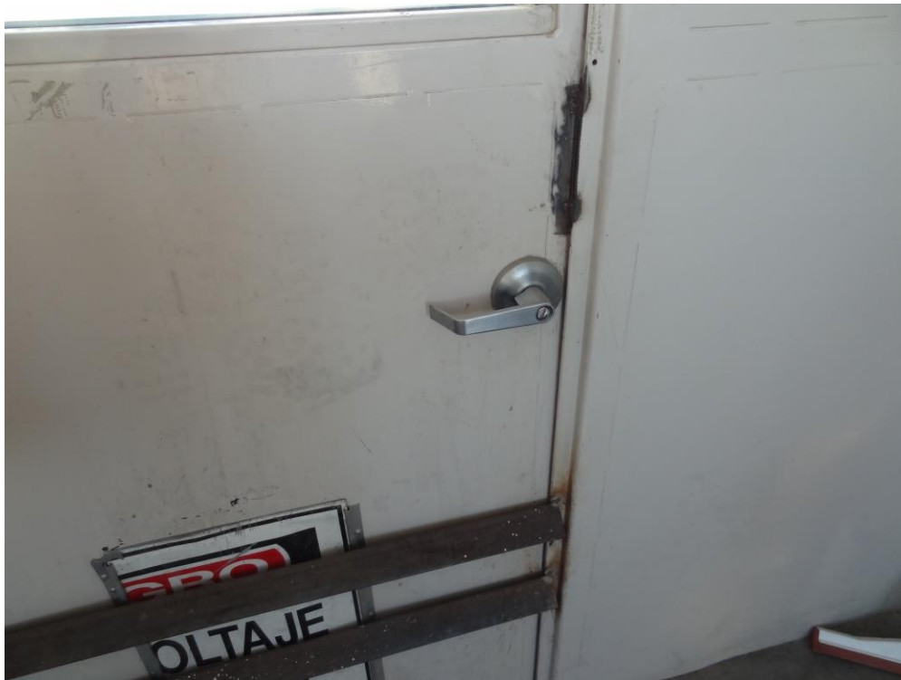
Sallyport - Building #2096 Description: Egress door upgrade needed.
