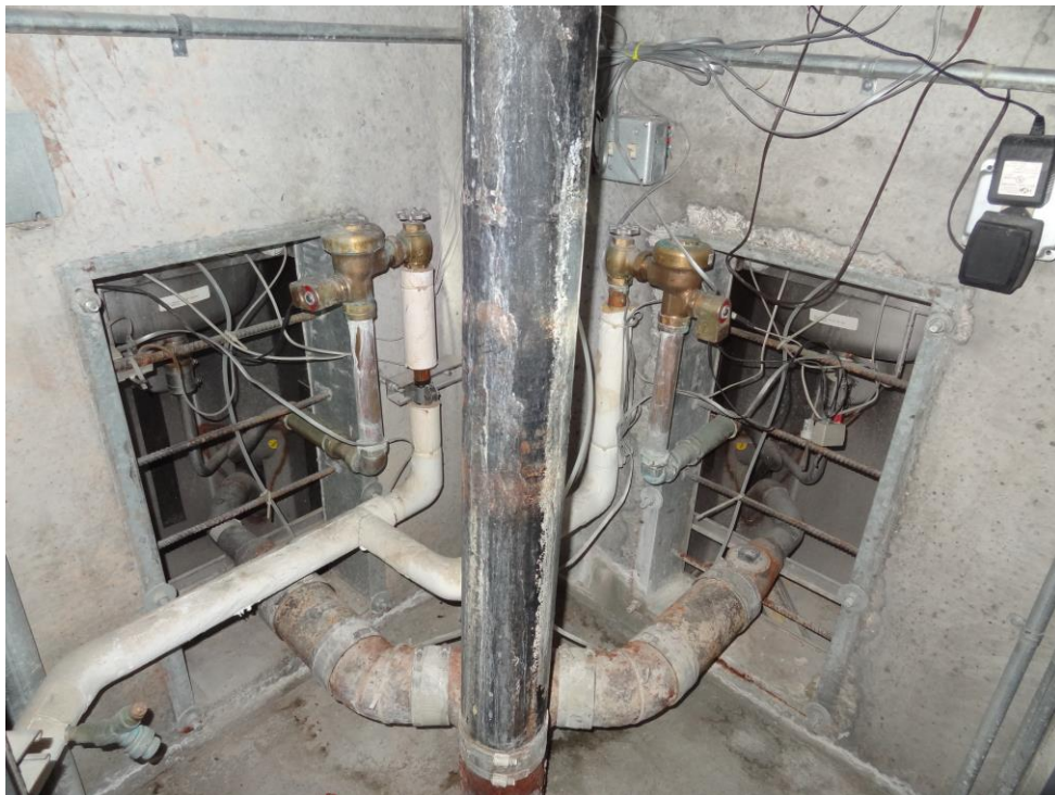
Housing Unit #7 – Building #2173 Description: Cell water controls system replacement needed.
