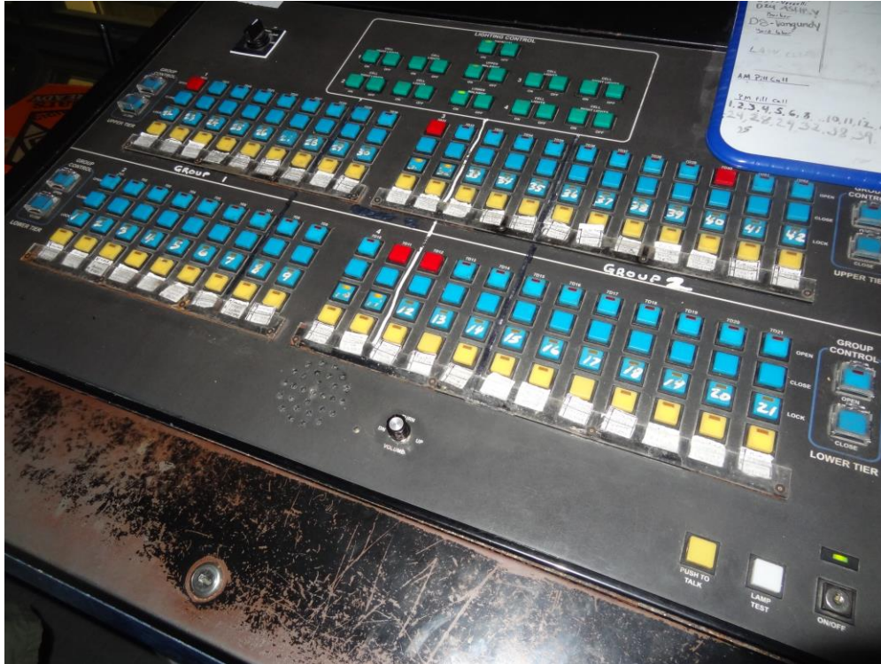
Housing Unit #7 - Building #2173 Description: Door controls system replacement needed.
