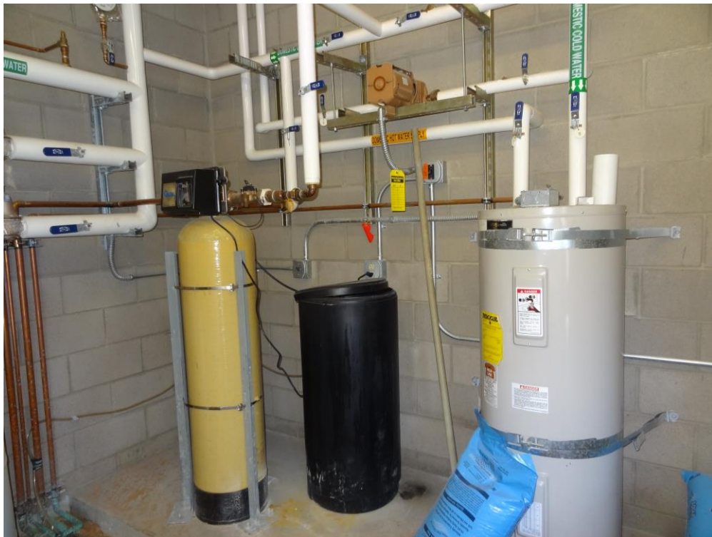
Security/ Administration - Building #2099 Description: Water heater replacement needed.
