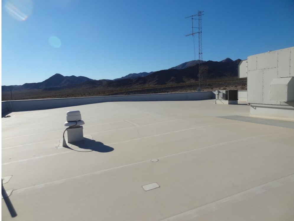
Administration - Building #2094 Description: Roof replacement needed.
