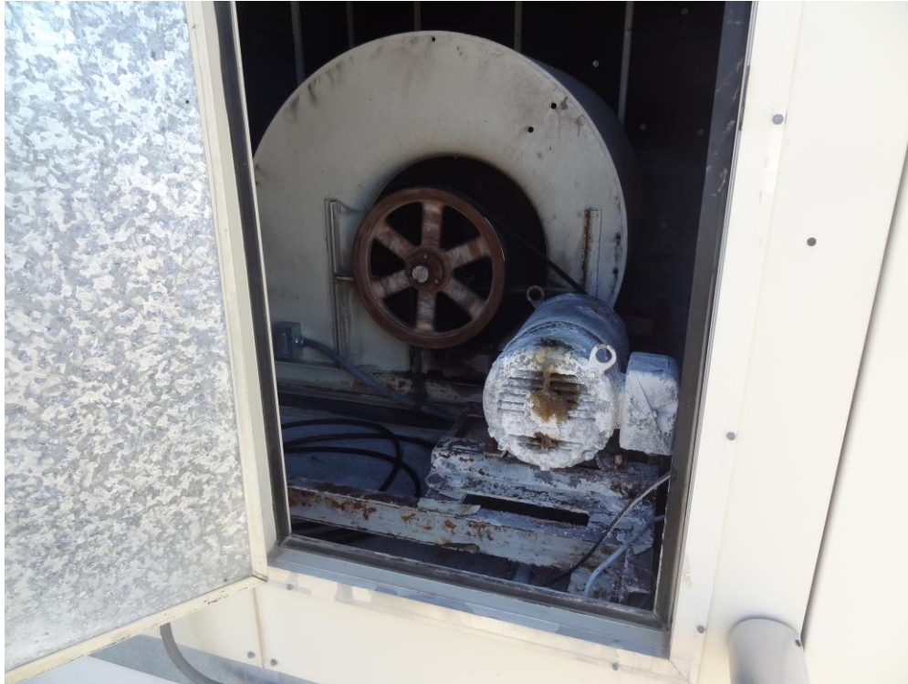
Maintenance/ Central Plant - Building #2097 Description: HVAC replacement needed.
