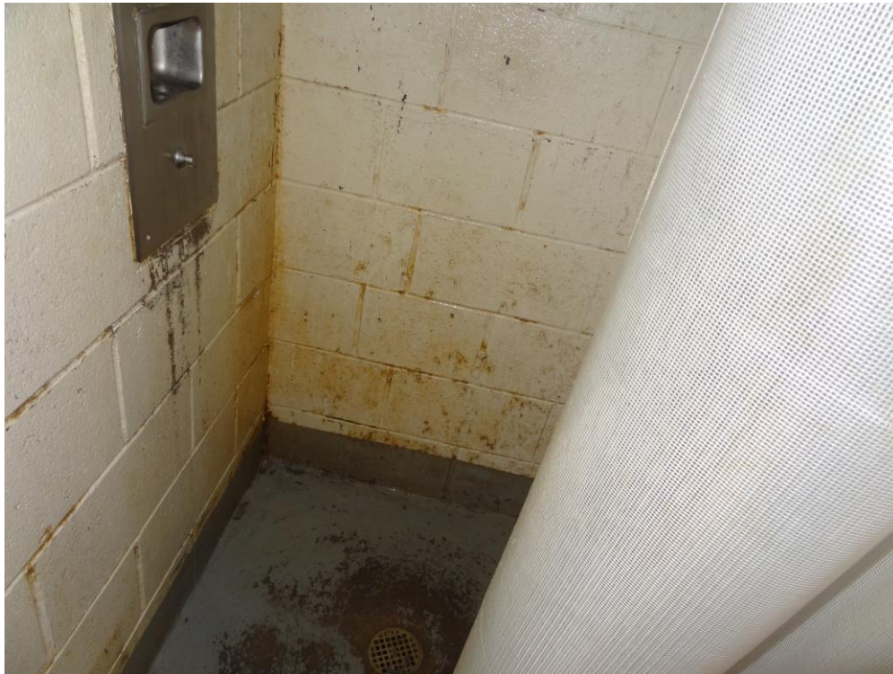
Infirmery/ Intake – Building #2090 Description: ADA shower upgrade needed.
