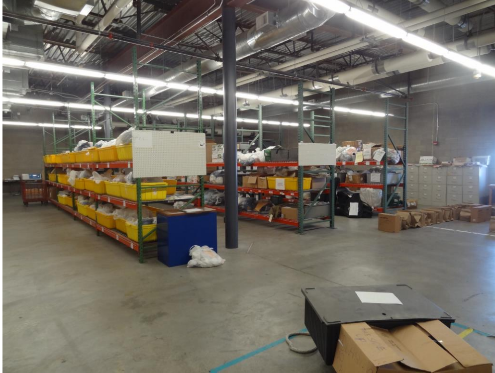
Infirmery/ Intake – Building #2090 Description: Shelves missing proper anchoring.
