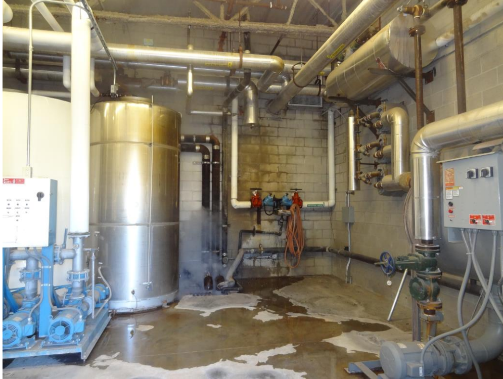
Inmate Services/ Culinary/ Dining - Building #2091 Description: Hot water re-use room remodel needed.
