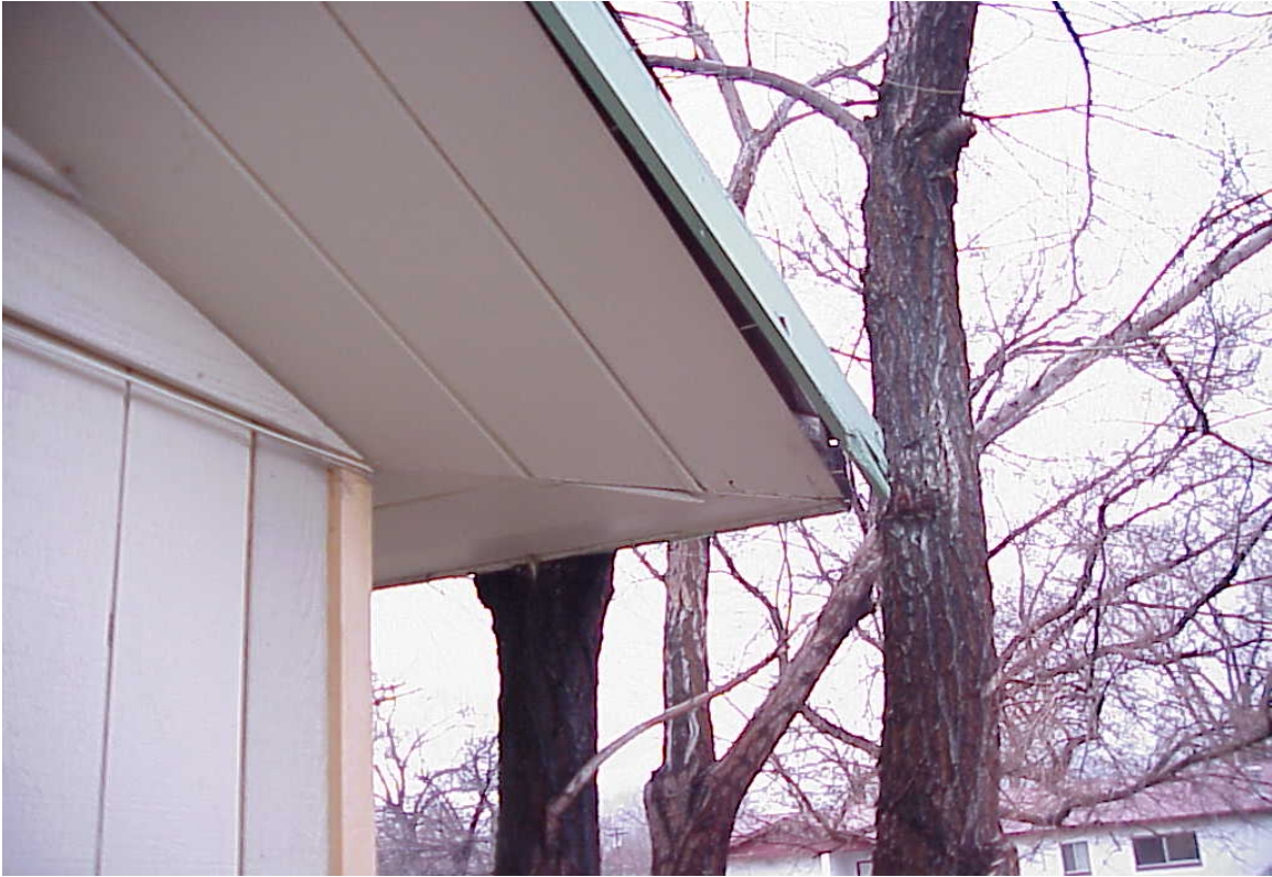
Child & Family Serv. Division/Boys & Girls Club/Hispanic Services - Building #0303 Description: Tree damaging the overhand of building.
