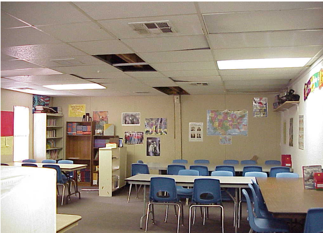
Child & Family Services Division/Education Center - Building #2309 1,650 square feet Description: The interior of the building with ceiling damage.
