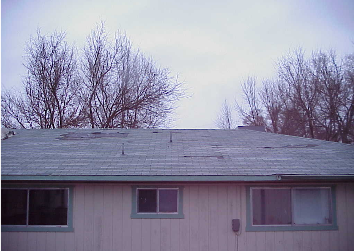
Child & Family Serv. Division/Boys & Girls Club/Hispanic Services - Building #0303 Description: Roof shingles missing, exterior of building.
