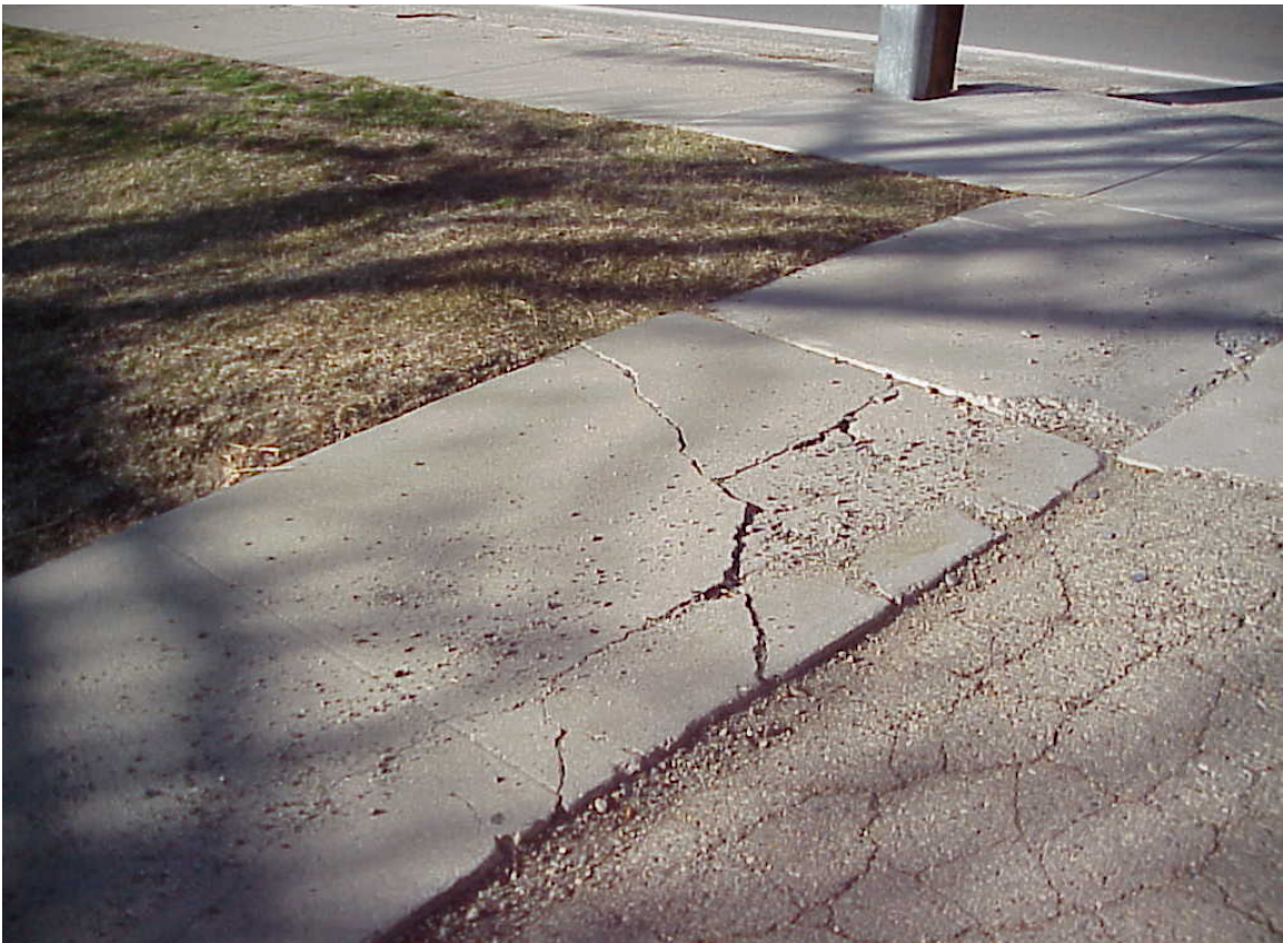
Child & Family Services Division Site #9955 Description: Typical sidewalk condition.
