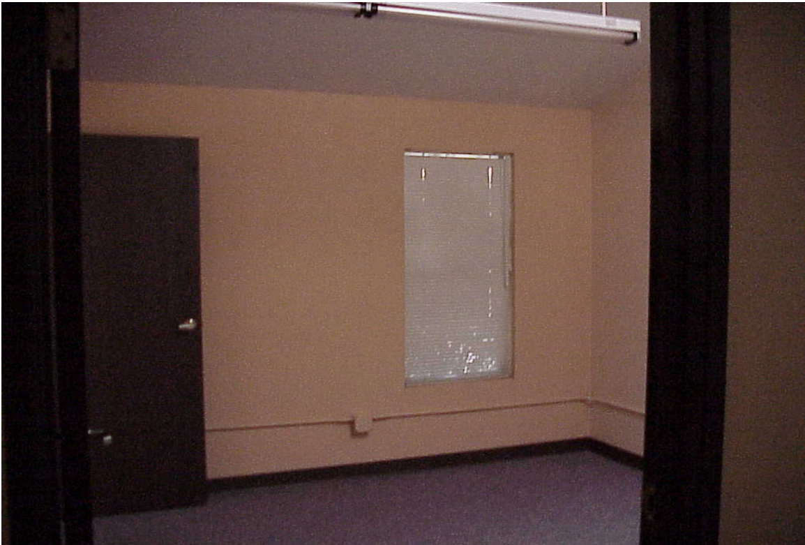
Child & Family Services Division/Rehabilitation Building (Vacant) - Building #0297 Description: Typical office space in building.
