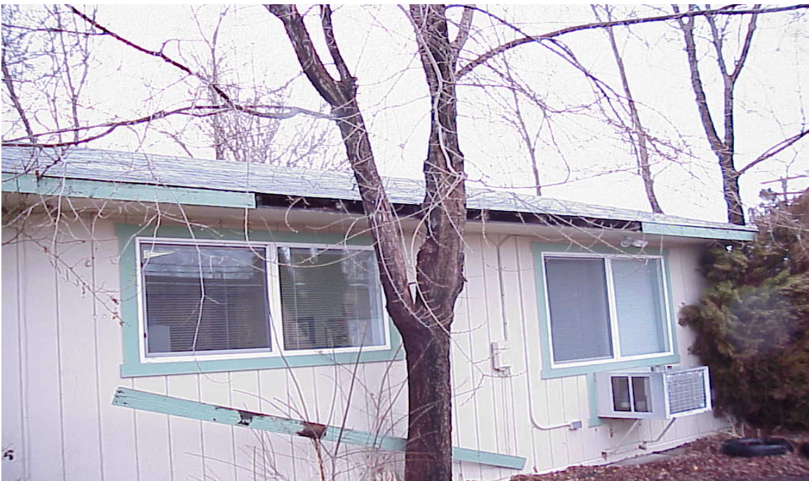
Child & Family Serv. Division/Boys & Girls Club/Hispanic Services - Building #0303 Description: Wind damage, exterior of building.
