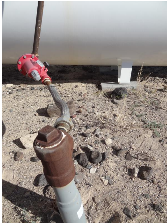
Tonopah Conservation Camp - Site #9975 Description: Gas line service needed.
