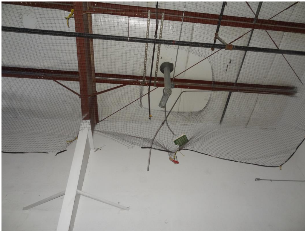
Multi-Purpose - Building #1619 Description: Heater replacement needed.
