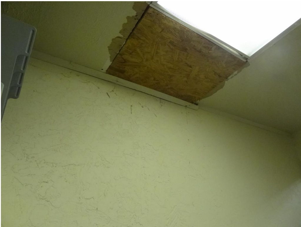
NDF Administration - Building #1620 Description: Fire rated ceiling repairs needed.
