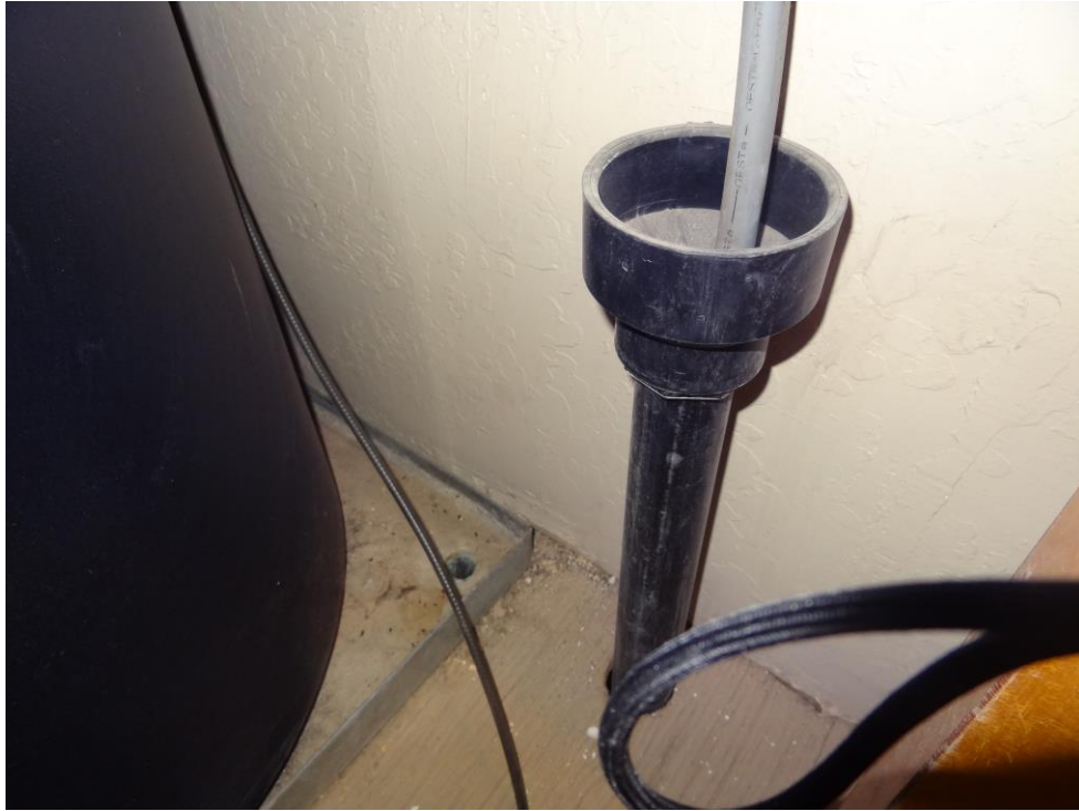
Multi-Purpose - Building #1619 Description: Plumbing replacement needed.
