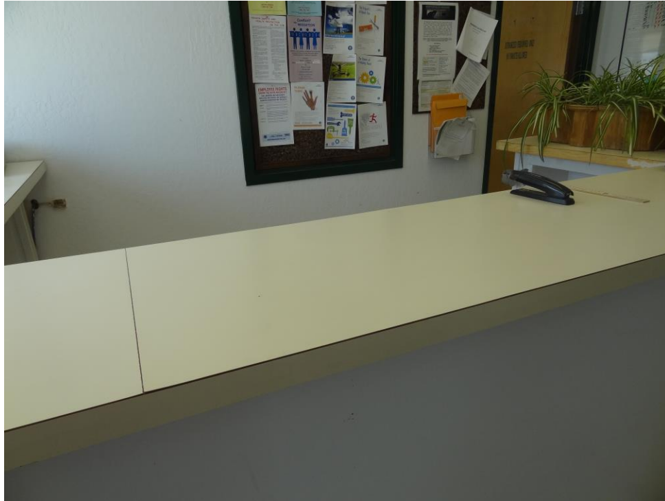
NDF Administration - Building #1620 Description: ADA accessible counter needed.
