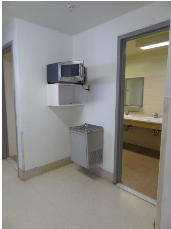
Housing Culinary Unit - Building #1618 Description: Dedicated circuits needed for microwaves.
