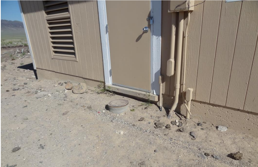
Pump House - Building #1621 Description: Exterior landing needed.
