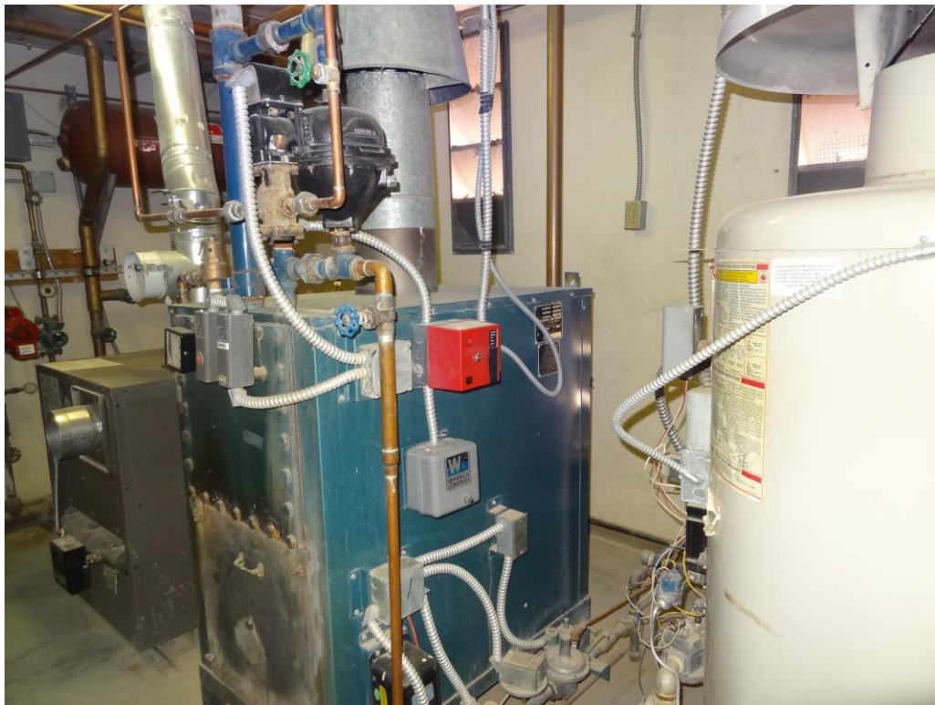
Housing Culinary Unit - Building #1618 Description: Boilers and heating system renovation needed.
