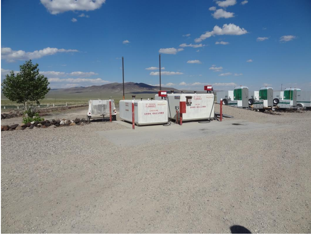
Tonopah Conservation Camp - Site #9975 Description: Site bollards needed.
