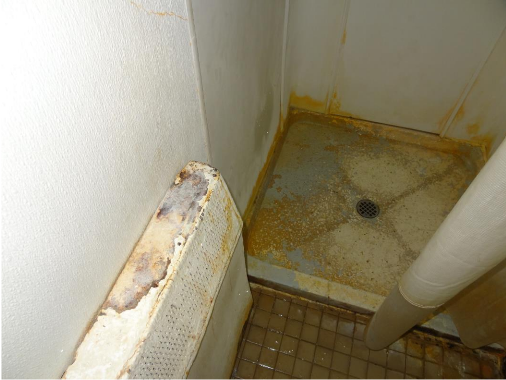
Housing Culinary Unit - Building #1618 Description: ADA restroom remodel needed.
