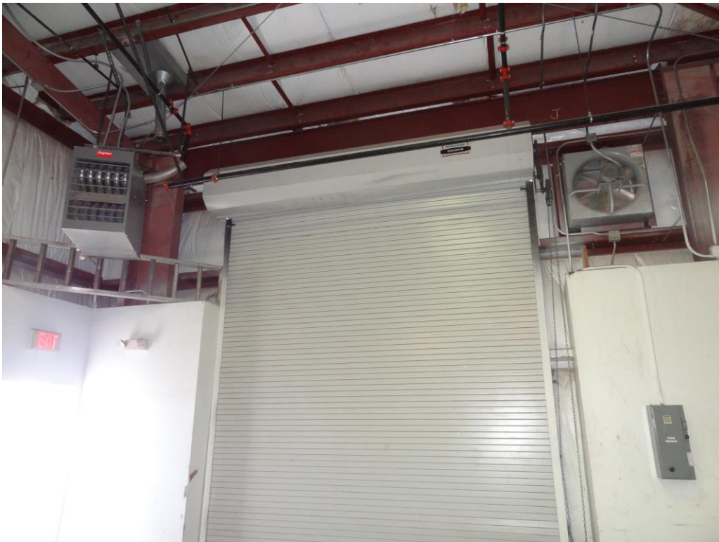
NDF Industry Building - Building #2493 Description: Flue replacement needed.
