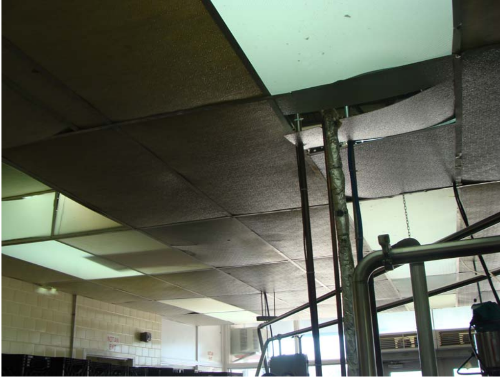
Dairy Barn - Building #1443 Description: Processing room ceiling in need of replacement.
