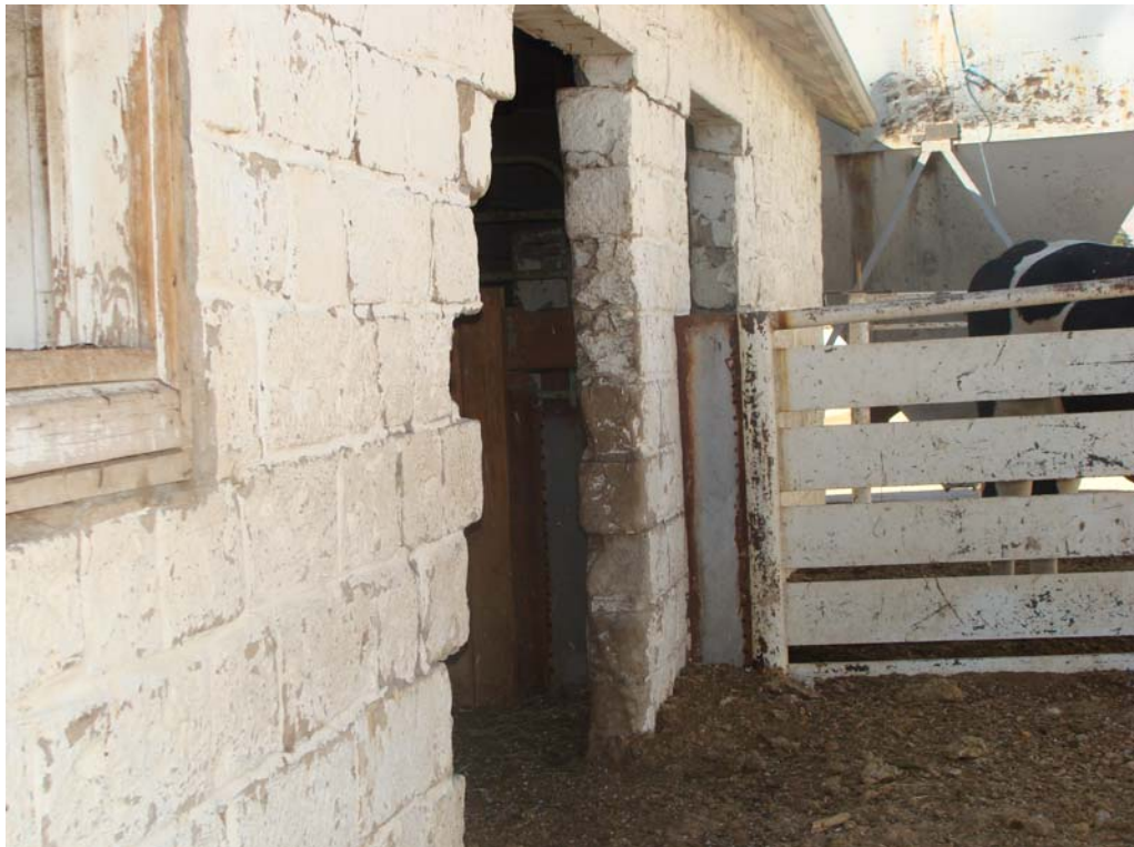
Bull Barn - Building #1440 Description: Exterior of the building, note structural wall damage.
