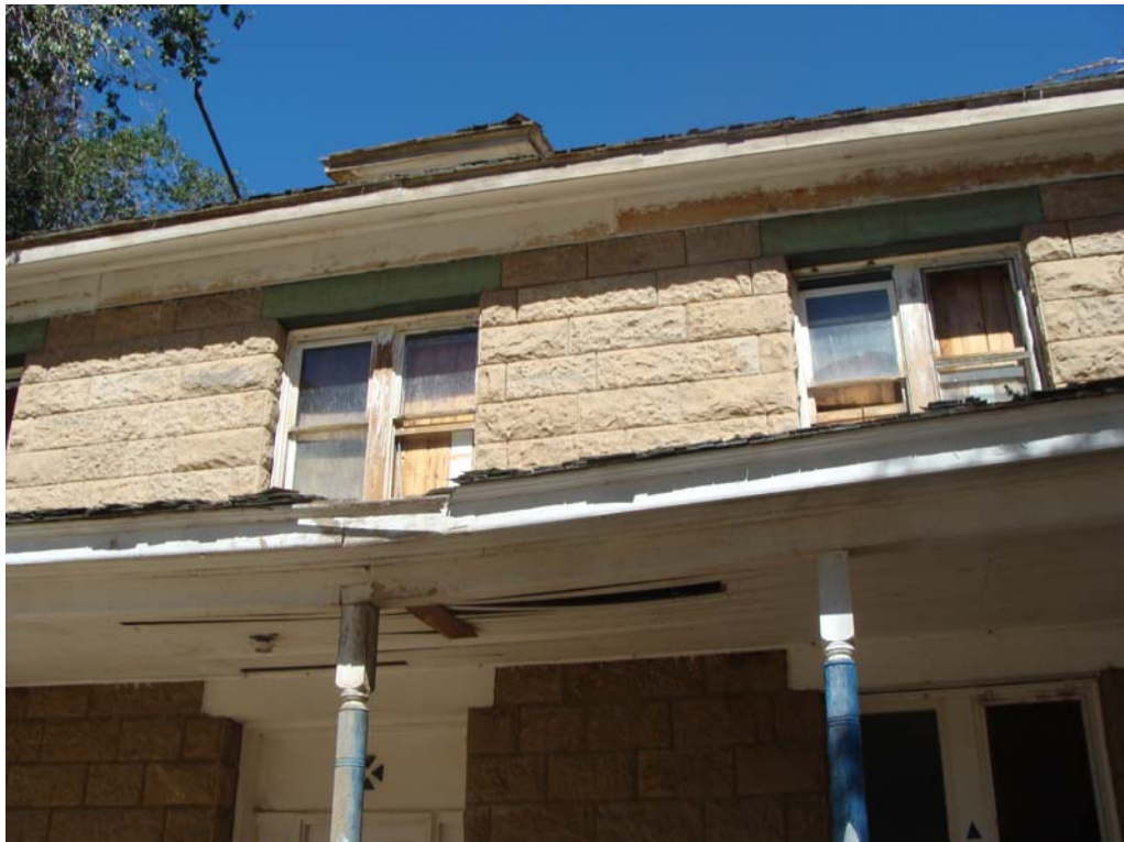
Ranch House - Building #1448 Description: Shed roof structural failure.
