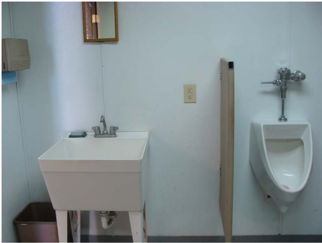
Maintenance Shop - Building #2915 Description: Non-ADA compliant restroom.
