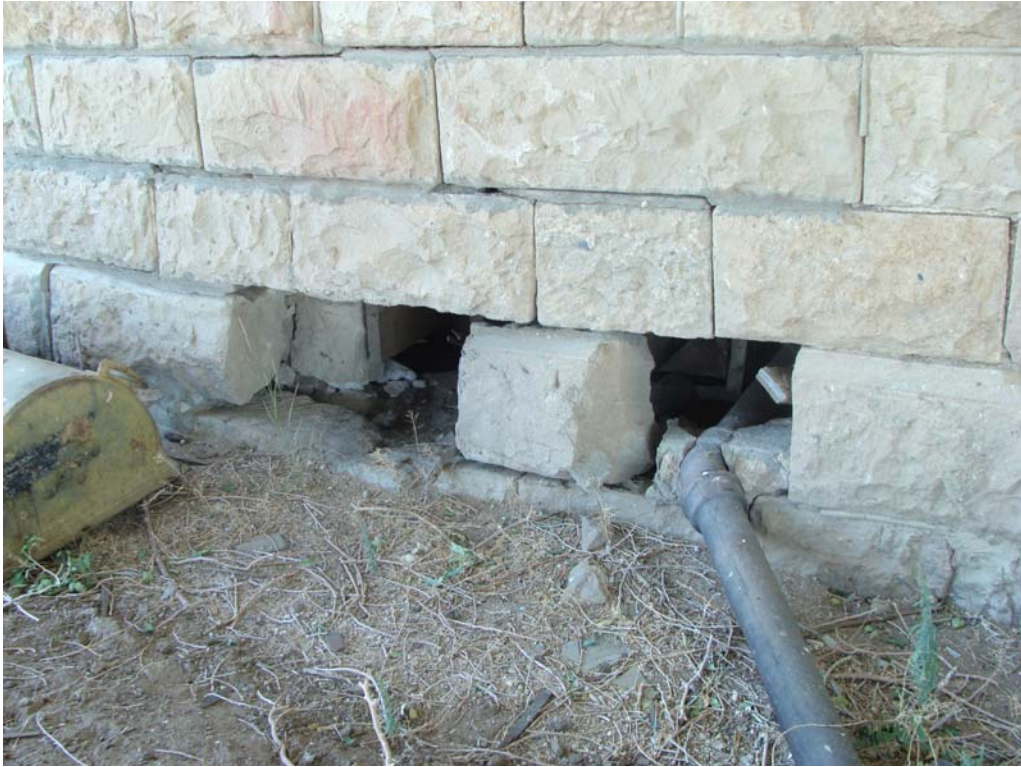
Ranch House - Building #1448 Description: Structural wall failure at foundation.
