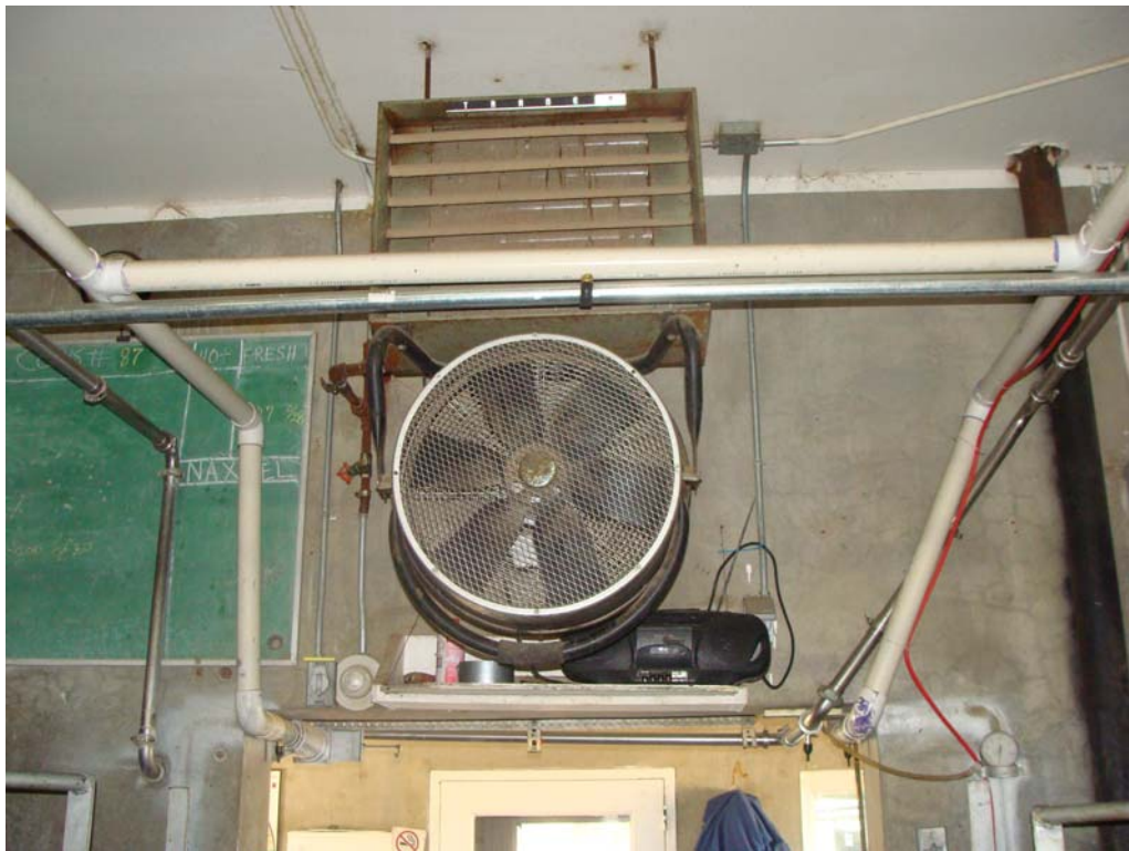
Dairy Barn - Building #1443 Description: Ceiling mounted heater in the milking area.
