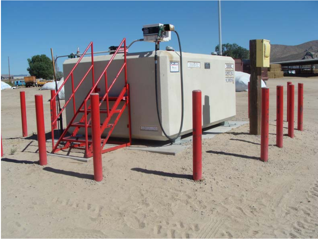
Northern Nevada Dairy Farm - Site #9982 Description: Above ground fuel tank.
