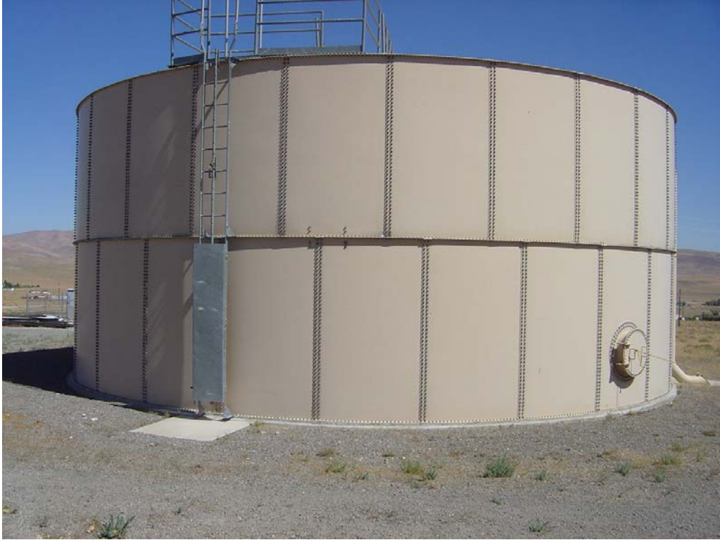
Silver Springs C.C. – Building #2690 Description: Water Tower
