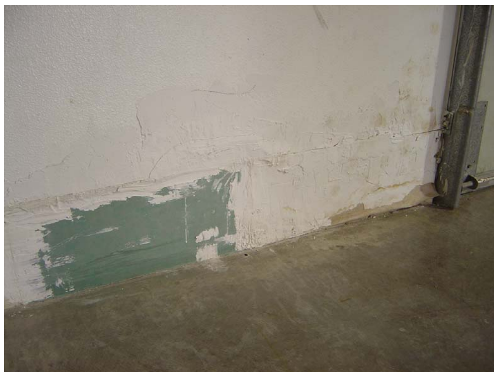
Silver Springs C.C. – Building #1896 Description: Gypsum board damage by overhead door
