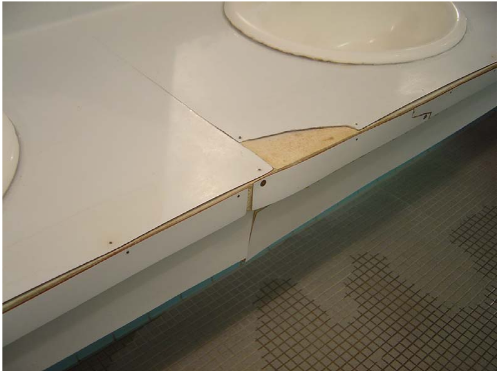
Silver Springs C.C. – Building #0711 Description: Typical damage to countertops
