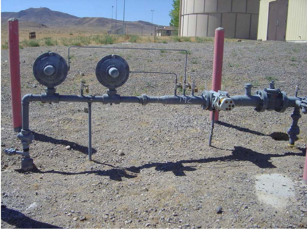
Silver Springs C.C. – Site #9986 Description: Gas main without seismic shut off valve
