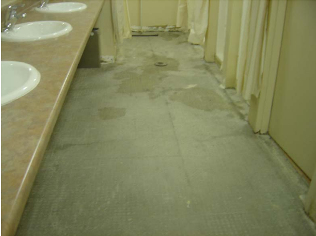
Silver Springs C.C. – Building #0711 Description: One of several floor drains with clogging issues
