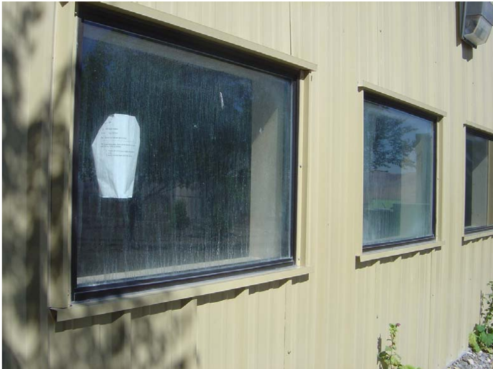
Silver Springs C.C. – Building #1895 Description: Windows in need of replacement
