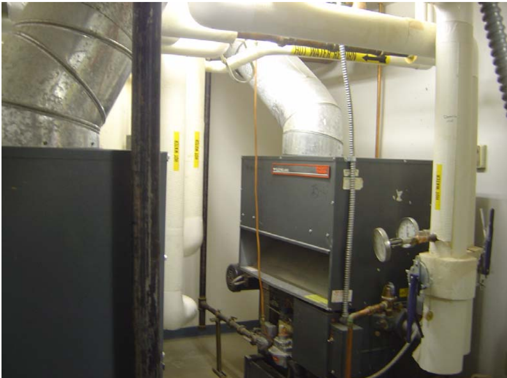
Silver Springs C.C. – Building #0711 Description: The Boiler Room
