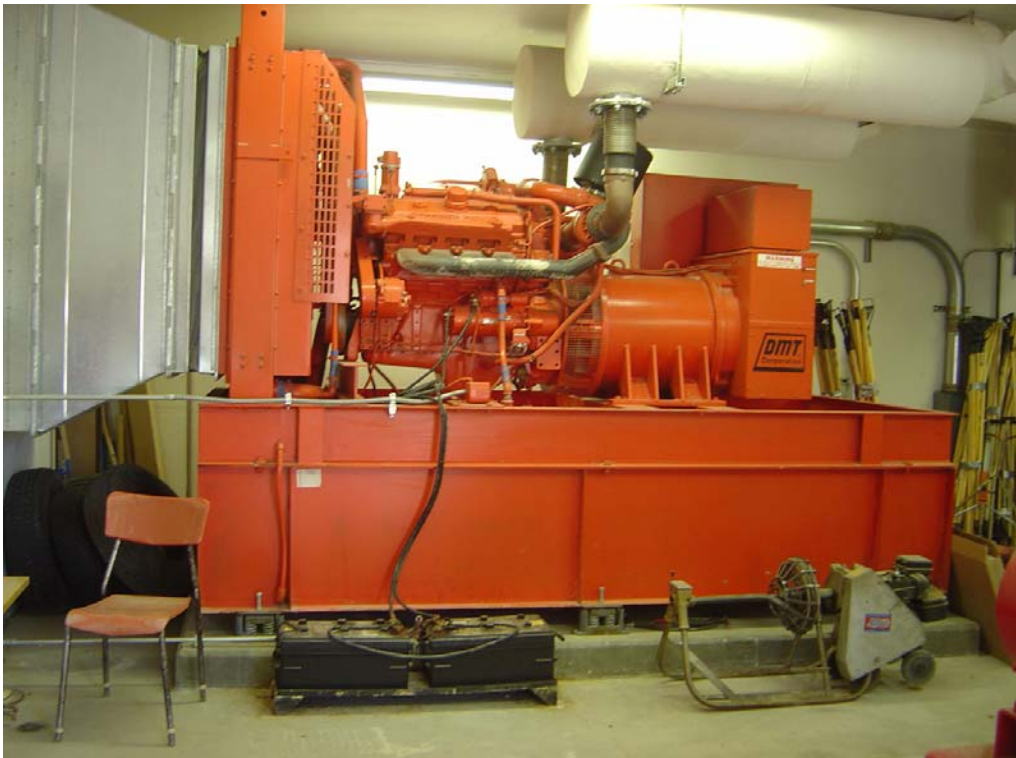
Silver Springs C.C. – Building #2029 Description: Generator
