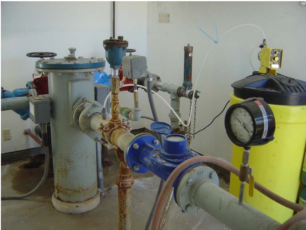
Silver Springs C.C. – Building #1352 Description: The interior of the Well House
