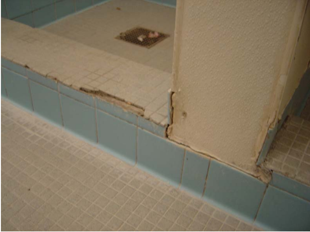
Silver Springs C.C. – Building #0711 Description: Damage to the showers, typical
