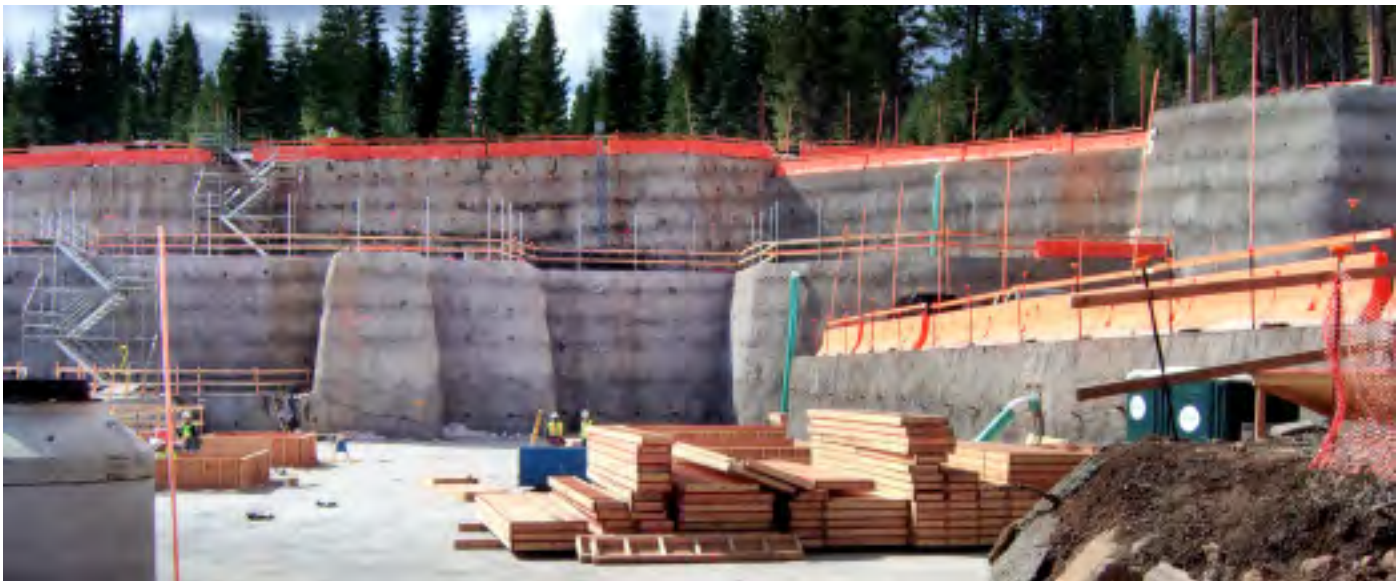
Above: A view of excavation and shoring at the Ritz-Carlton Lake Tahoe, where 40-foot-high retaining walls were required - see personnel in photos and multi-tiered stairs for scale.
